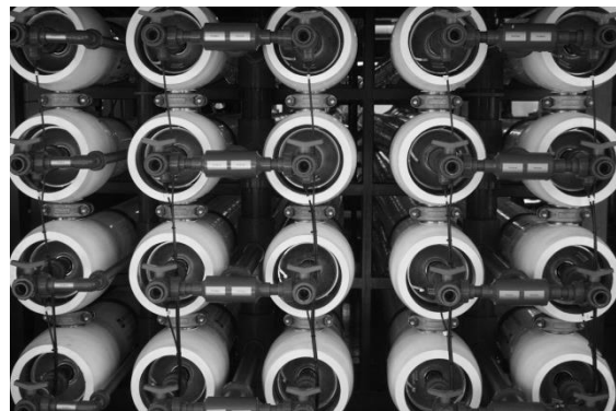
fig. 74 Arrangement of Reverse Osmosis Tubes
