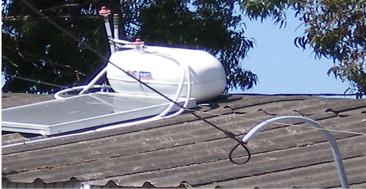
Photo 2: solar water heater on the roof of council built house in Zwelitsha (80L system)
