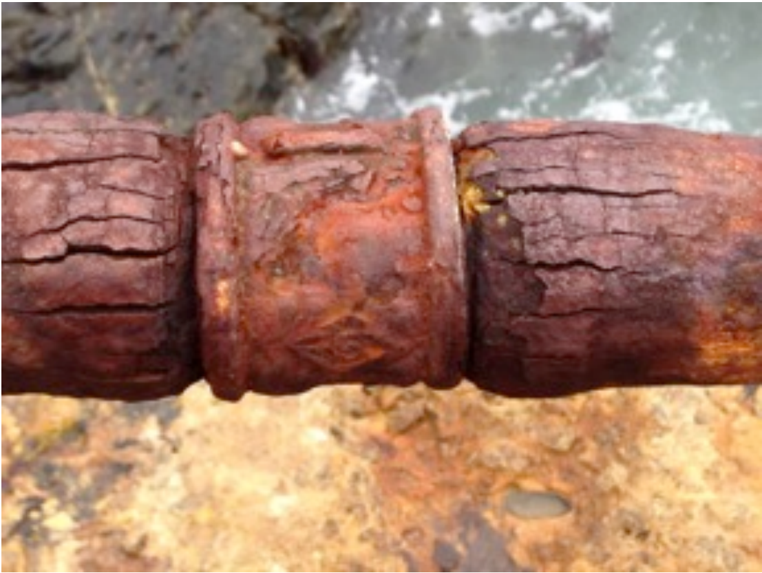
Figure 2. Rusted handrail Cape Town, South Africa. Photo credit to Janis Milligan 2014.
