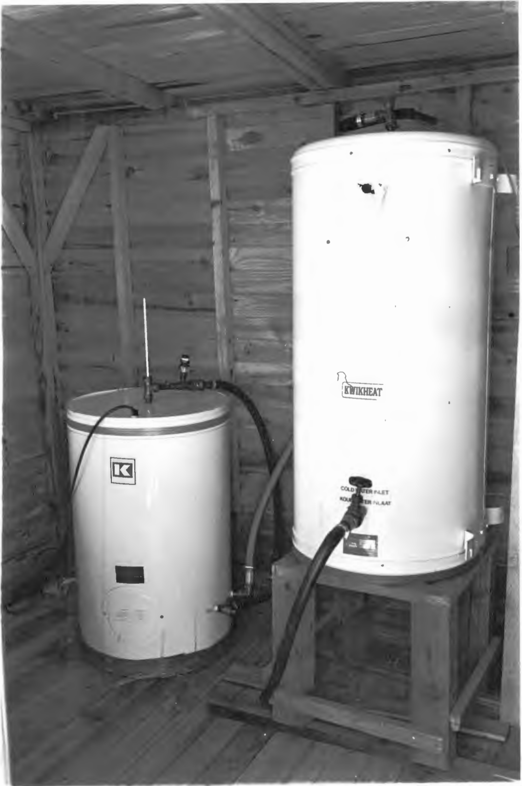
Figure 5.1.3 The Storage Tanks
