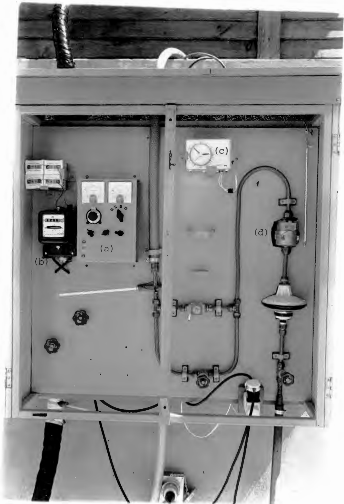
Figure 5.1.4 The Instrument Box (a) the thermistor circuit (b) the kWh meter (c) the timer clock (d) the water meter
