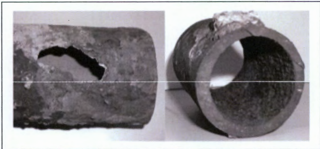
Figure 2-9: Cast Iron Pipe, Corrosion, Graphitisation and Incrustation ( (JM. Rodriguez, 2012)
