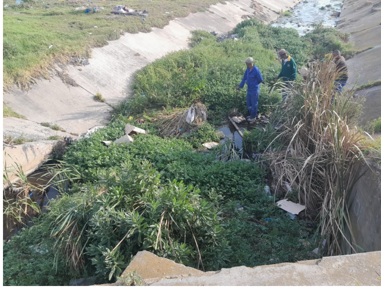
Figure 6-16: Overgrown channel and illegal litter dumping at Site 14 (Bethelsdorp) (September 2022)
