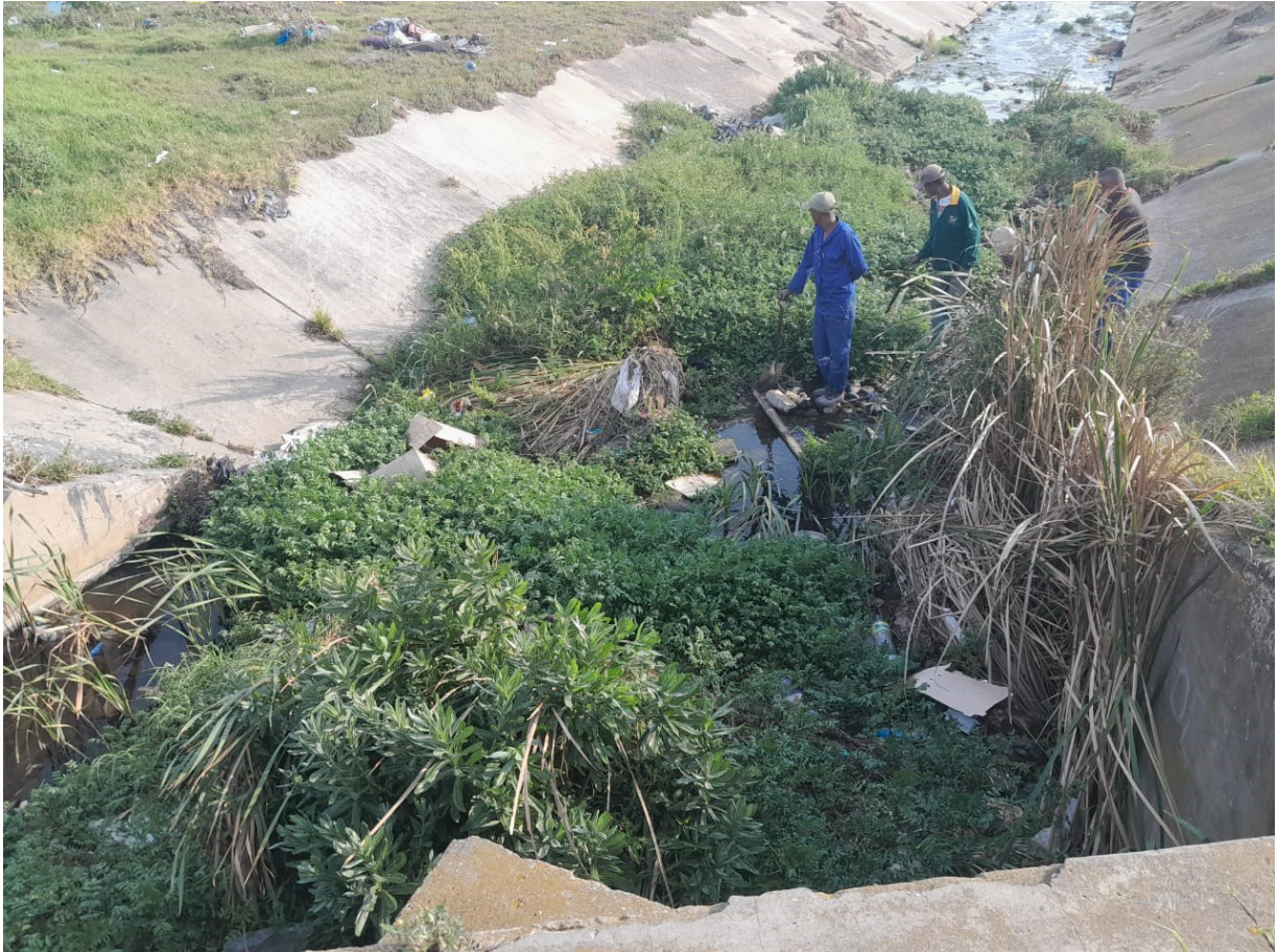
Figure D-4: Overgrown channel and illegal litter dumping at Site 14 (Bethelsdorp) (September 2022)
