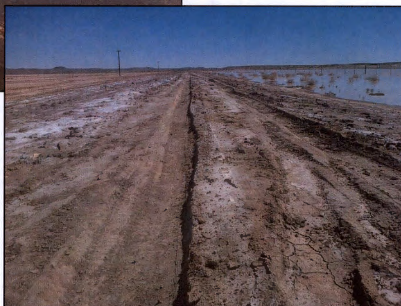
Figures 3.4a (top) and 3.4b (bottom) Photographs depicting the flooding and resulting degradation of gravel roads within the study area.
