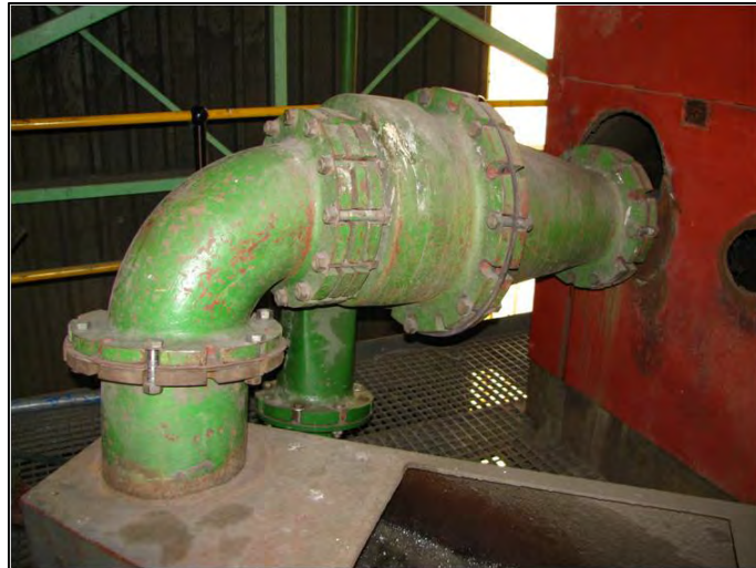
Figure 3.4 Dense medium cyclone at the Mintek pilot plant
