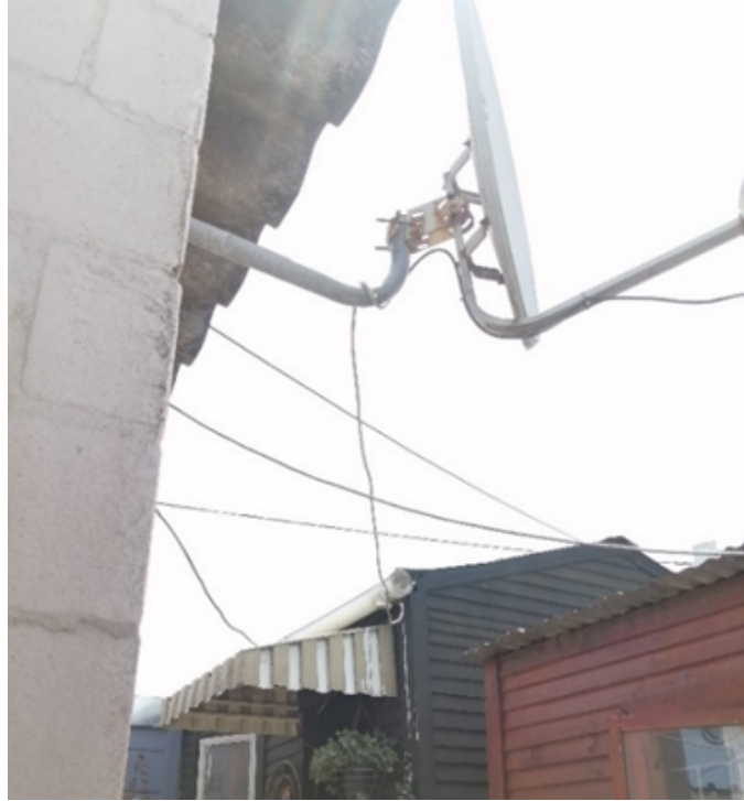
Image 25: Illegal electric connections. Source: Author (2022)
