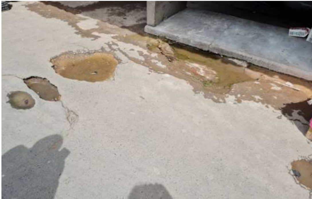
Figure 8 Potholes and Puddles in Warwick (Outside EMM).
