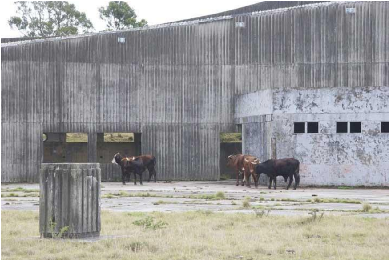
Figure 12 Empty concrete plinth where Sebe's bronze once stood in the centre of Ntaba kaNdoda monument. Nguni cows wander in the background. Photograph taken by William Martinson, 2014.
