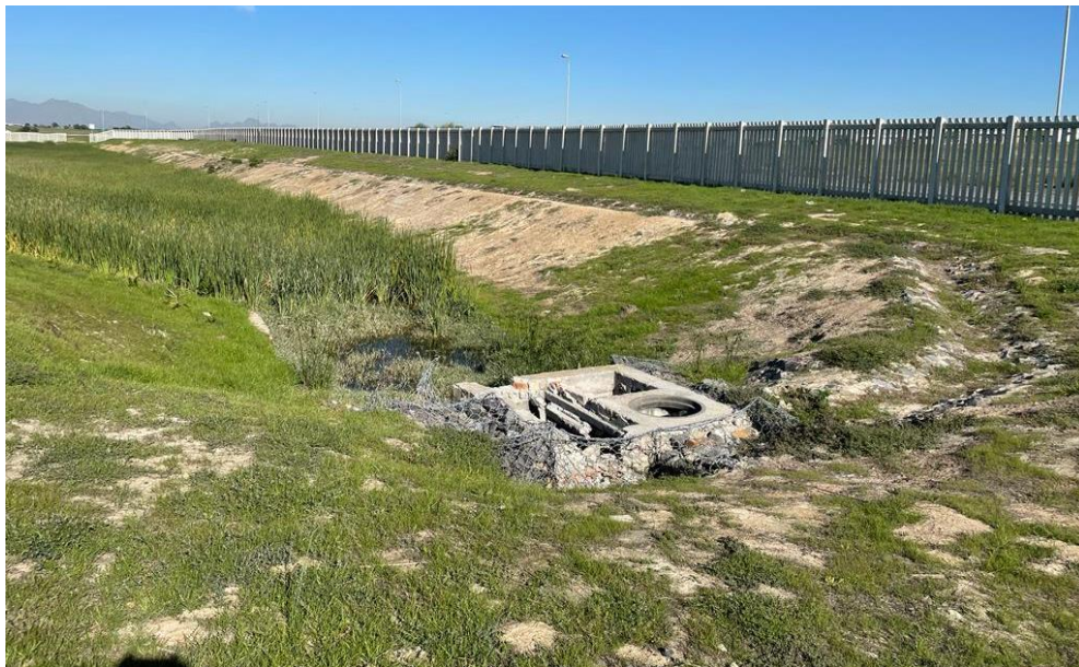
Figure 44: A vandalised inlet
