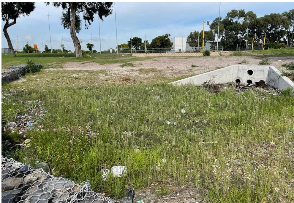
Figure 48: A detention pond inlet
