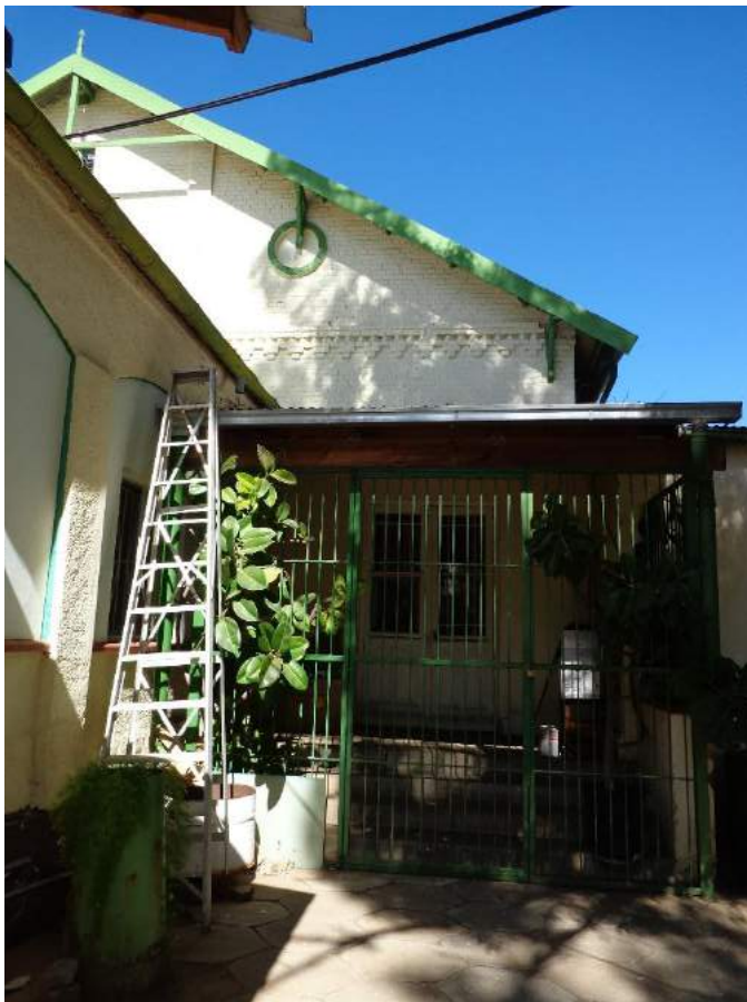
Figure 24 The original decorative timber gable finishing has disappeared, additions obscure part of the building (photograph by author, 21 July 2017)
