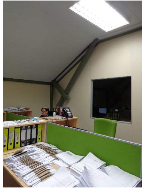
Figure 37 The original timber roof structure is visible in the suspended first floor office space which replaced the original double volume (photographs by author, 7 April 2017)
