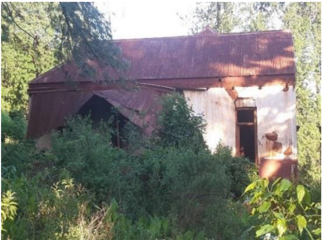
Figure 49: Dilapidated western wing of parsonage (Source: Author, 2014).
