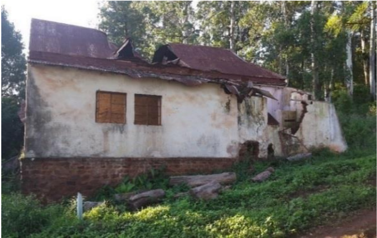
Figure 48: Dilapidated eastern wing of parsonage (Source: Author, 2017).
