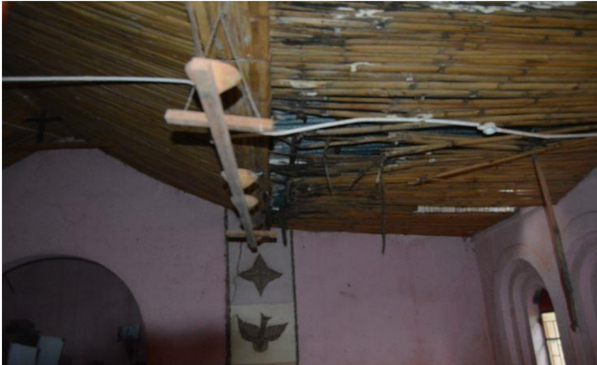
Figure 59: Bamboo ceiling damaged by rain water (Source: Author, 2017).
