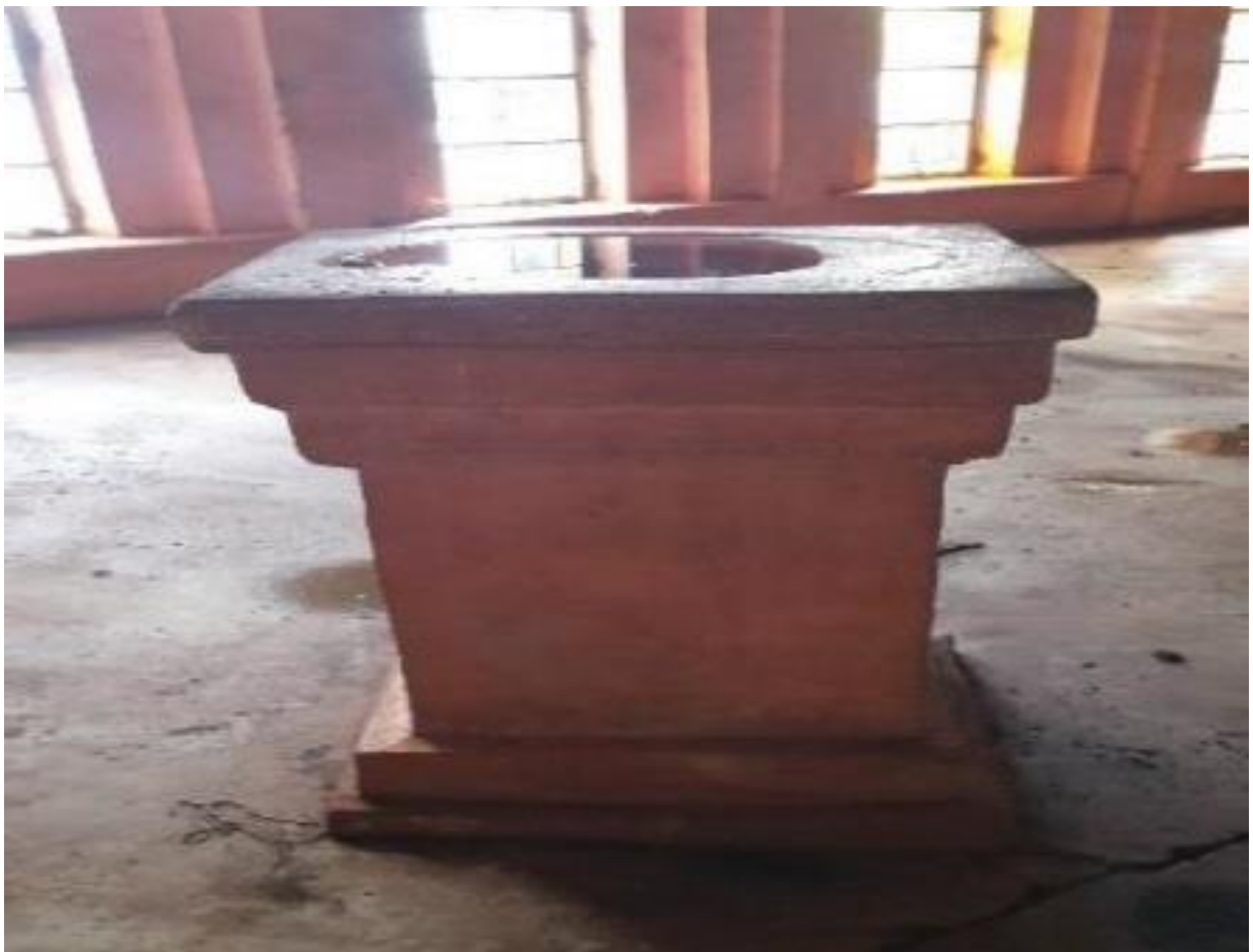
Figure 58: Baptismal font with rain water that leaked through the roof (Source: Author, 2014).
