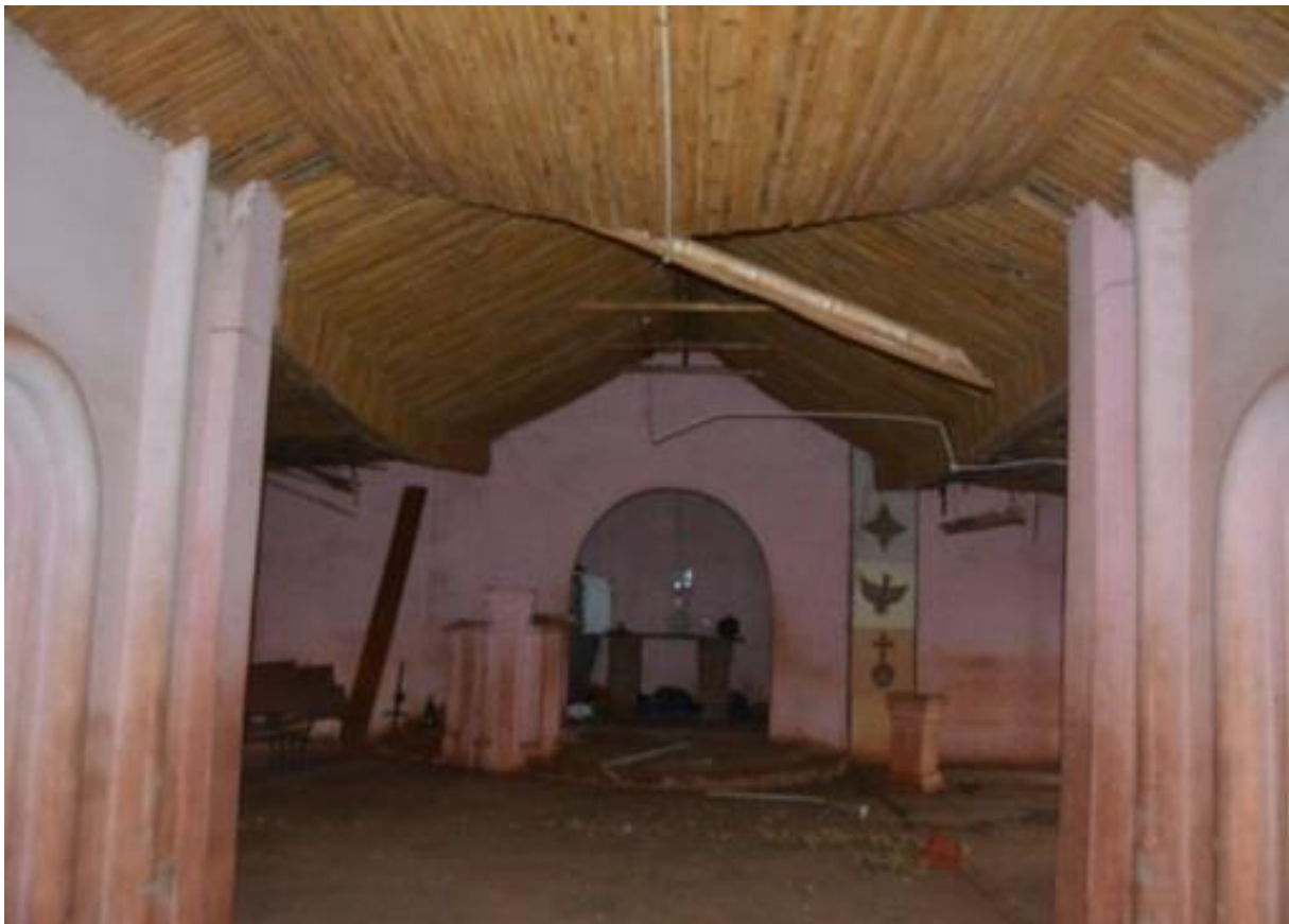
Figure 56: Poor state of neglected Church inside (Source: Author, 2017).
