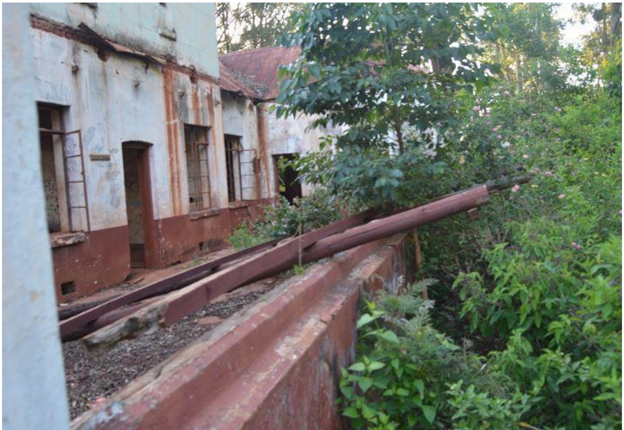
Figure 53: Fallen veranda roof at the back of parsonage (Source: Author, 2017).
