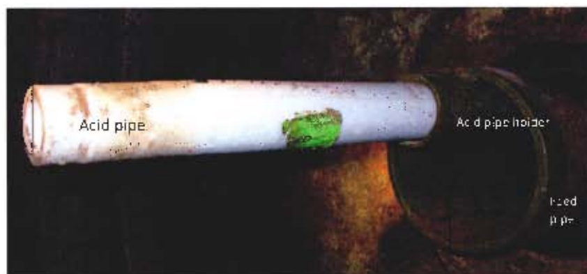
Figure 7: HAL mineral feed pipe and acid feed pipe
