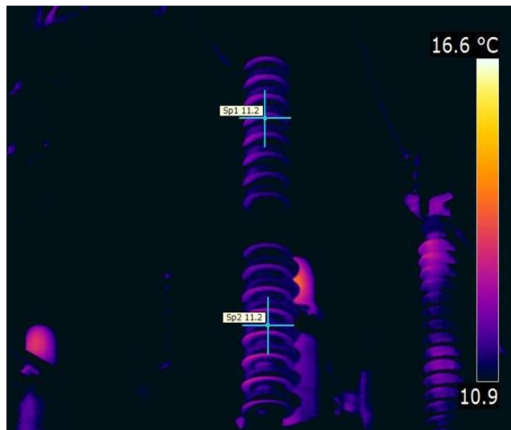
Figure D. 7 Thermal image of the Bloedrivier - Normandie red phase 88kV surge arrester
