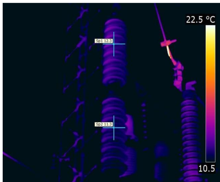
Figure D. 8 Thermal image of the Bloedrivier - Normandie white phase 88kV surge arrester
