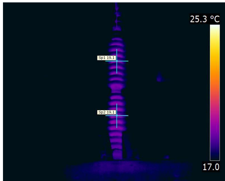
Figure D. 5 Thermal image of the Umfolozi – Bloedrivier white phase 88kV surge arrester
