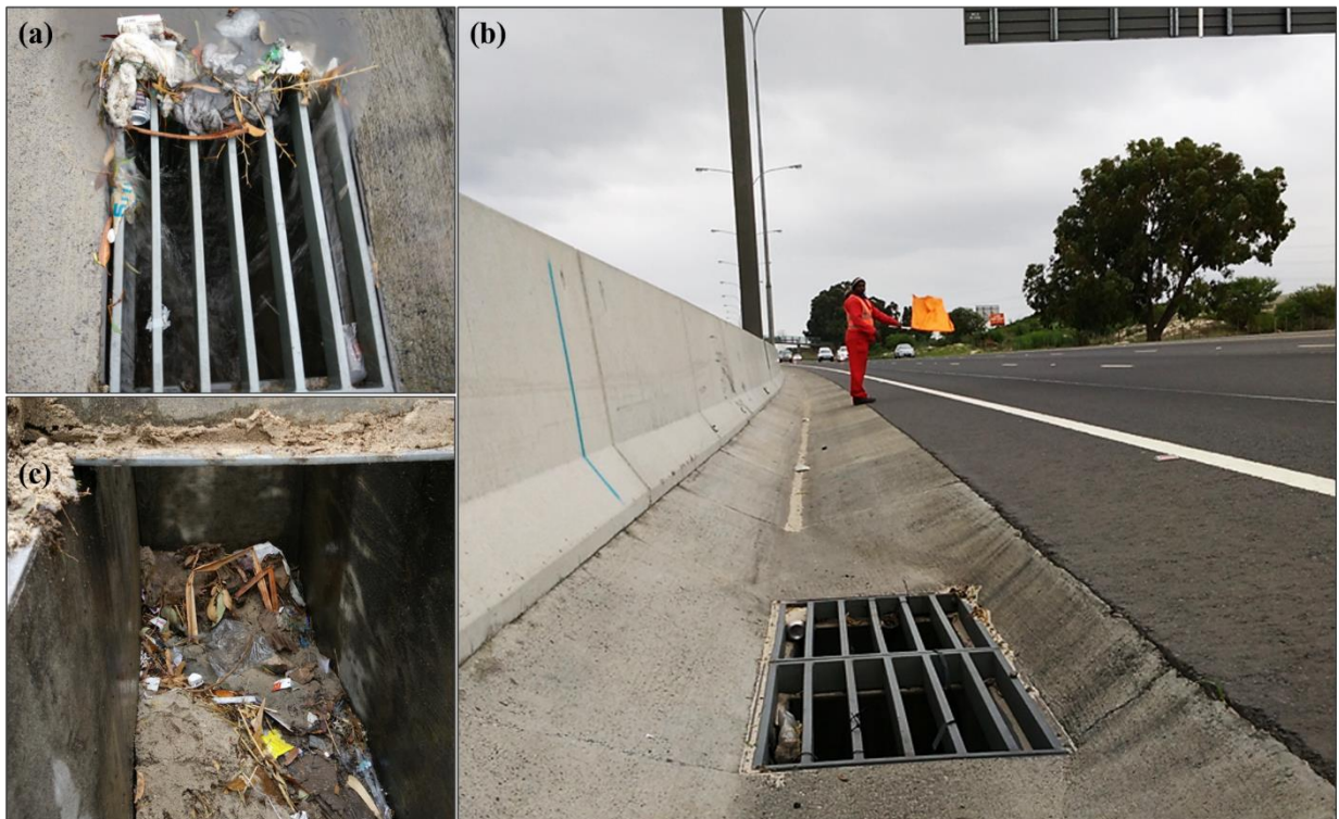
Figure 4-4: Sample Site 2 (a) the catchpit inlet grid, (b) the asphalt catchment and concrete median drain, and (c) view inside the catchpit
