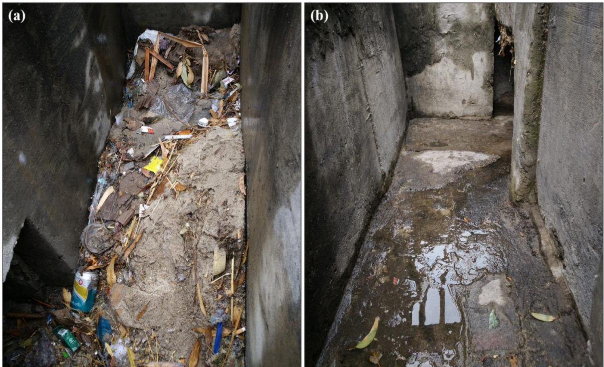
Figure 3-10: Median catchpit scoured clean by a rainfall event: (a) prior (b) subsequent to a rainfall event
