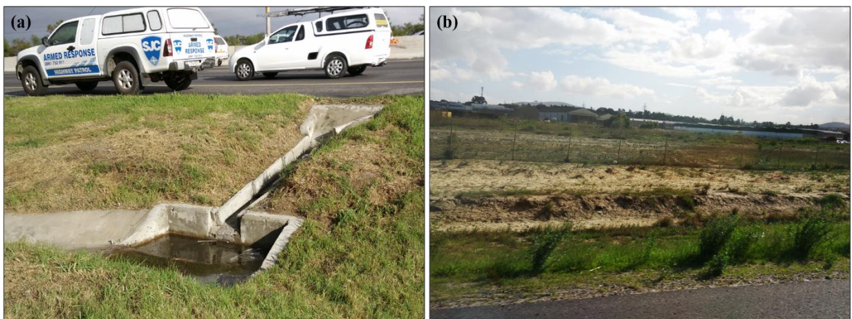
Figure 3-8: R300 road drainage structures located in the verge: (a) concrete down chute, and (b) sandy drainage ditch
