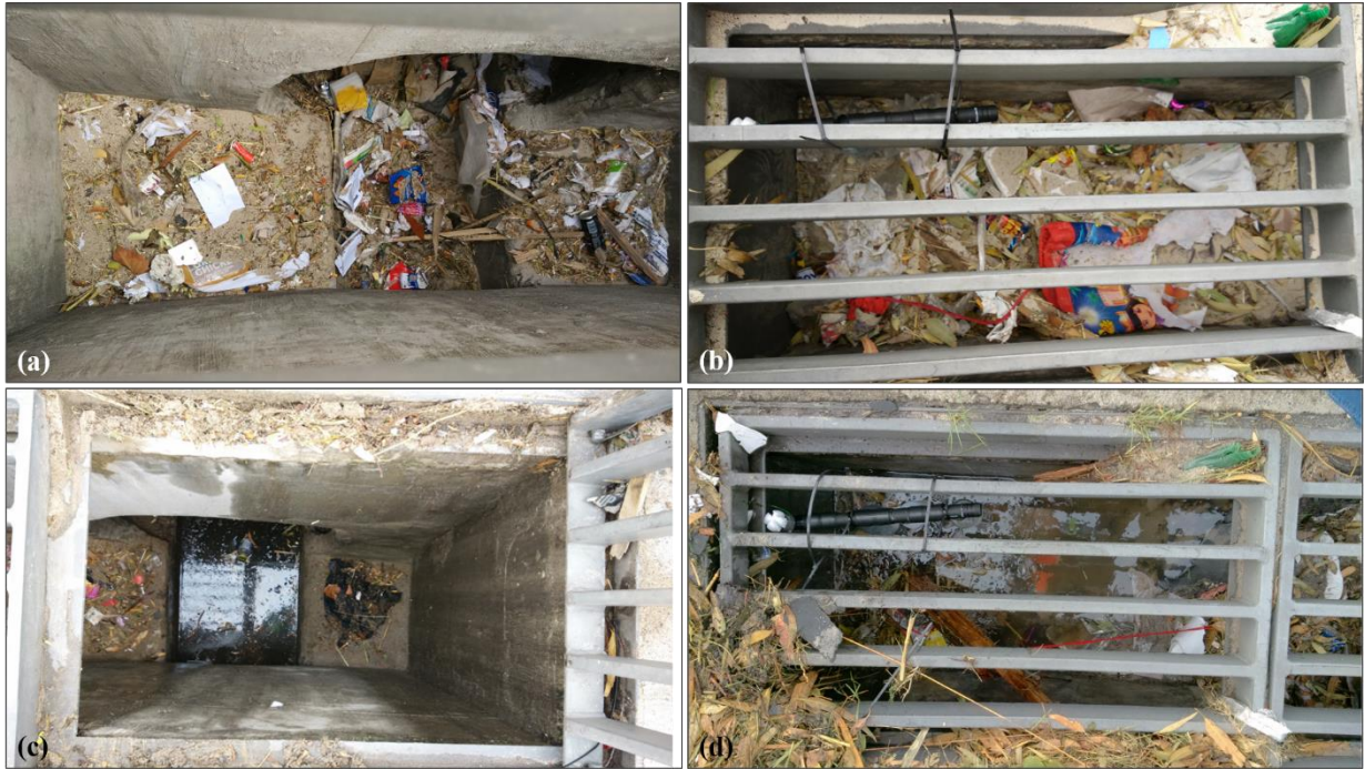
Figure 3-11: Accumulated solid waste in median catchpits: (a) food wrappers, cigarette butts and sediment, (b) packaging waste, (c) silted up drain, and (d) blocked drain
