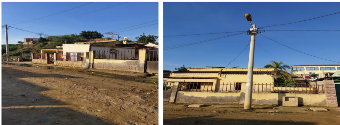
Figure 11: Unsafe electrical cables linked to a public utility pole, with stagnant water from the rainfall in front of a residence, posing a potential hazard to the residents. Photo credit: Ngoia de Lemos, 2024.
