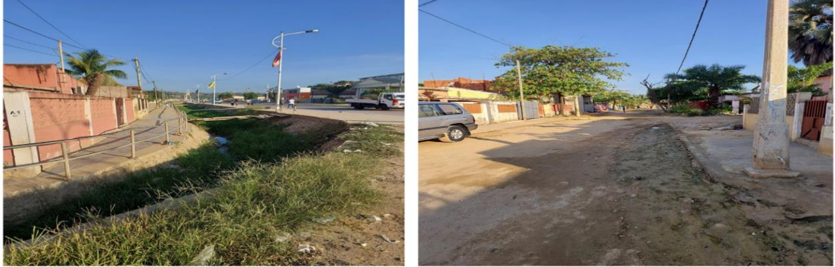
Figure 7: The drainage ditch in the Assaca neighbourhood floods during heavy rainfall. On the right is a representation of the many unpaved streets in the Assaca neighbourhood.
