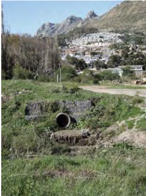
Stormwater pipe discharging effluent from Imizamo Yethu into the Hout Bay River
