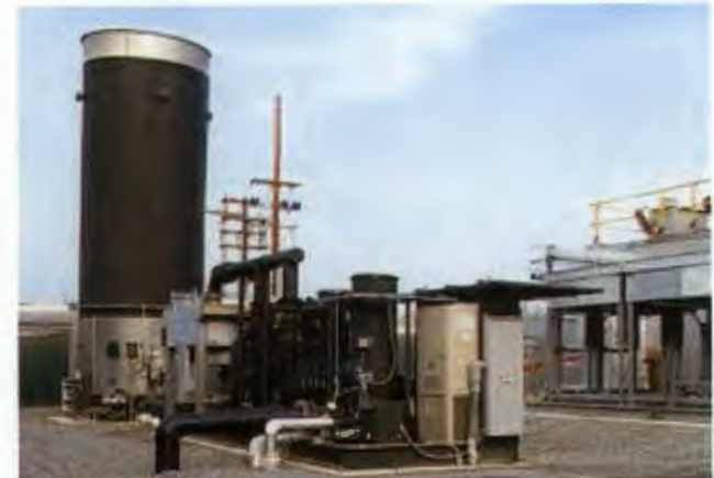
Fig 63 Fuel extraction tanks at the landfill
