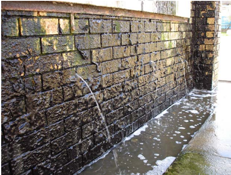
Figure 5.11: Leaking on the North face during the investigation period
