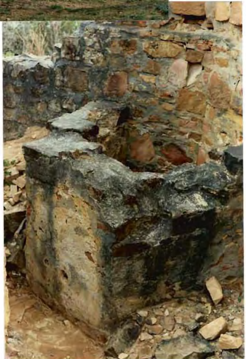
Fig. 195 Cistern inside the Blockhouse, 1993. Note the floor in front of the water outlet.
