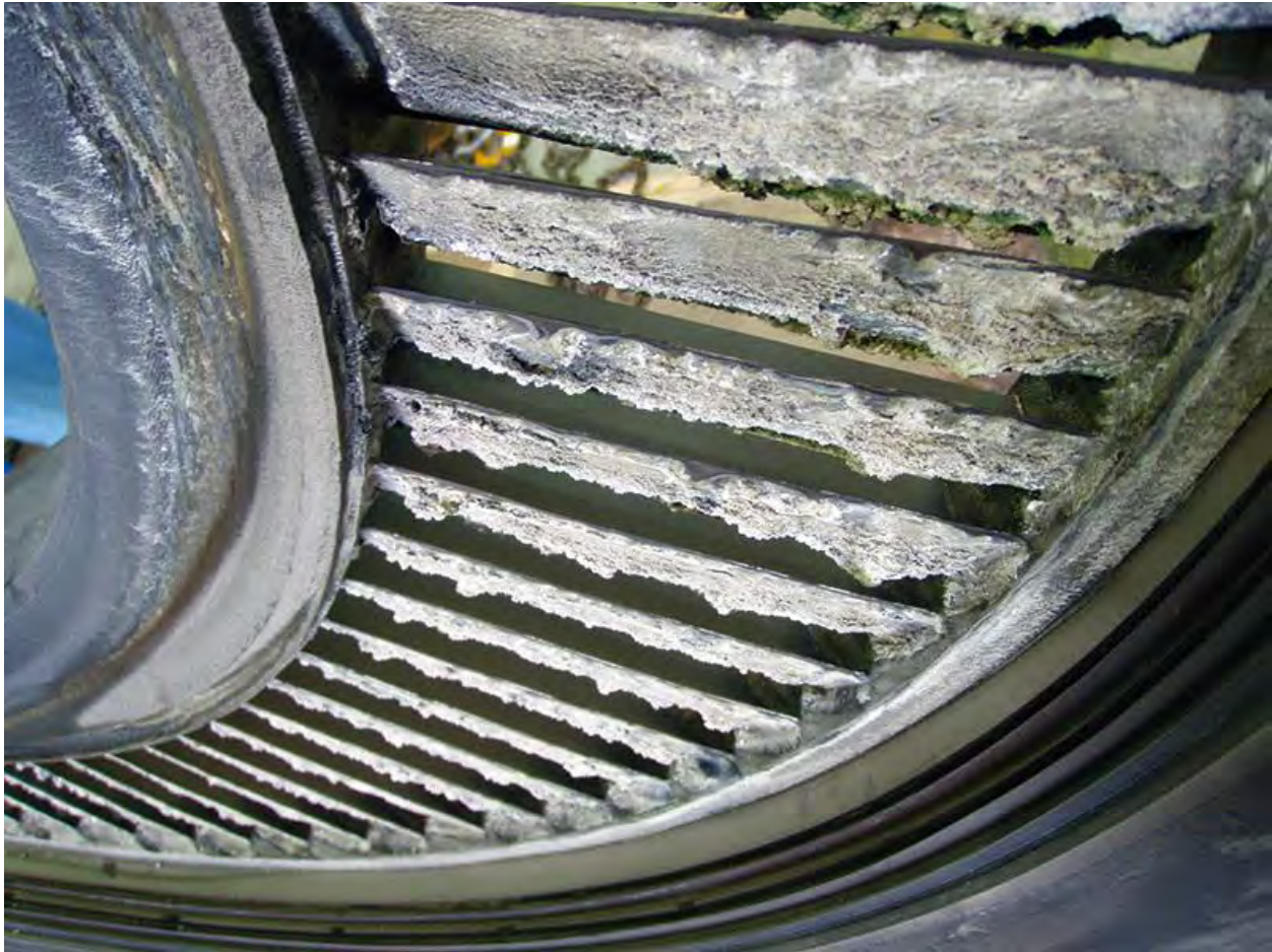
Figure 69. Scale formation on a turbine stator (Mitsubishi Heavy Industries, 2012).
