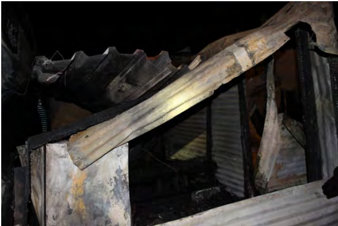
Figure 7: A burned, unstable and unsafe informal house in which remains were retrieved
