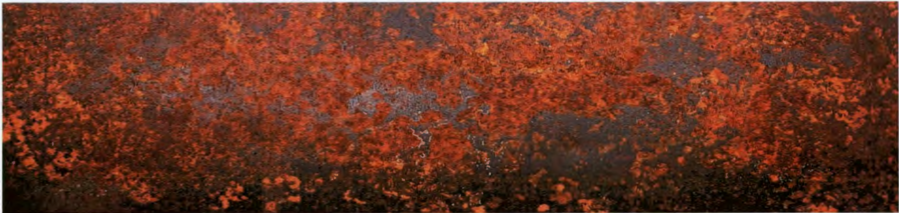
Image 15: Rust “Wall Art”
