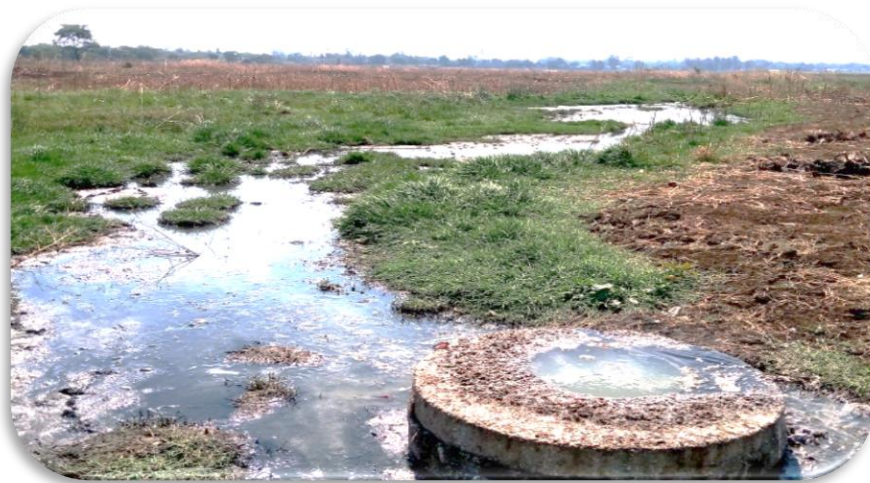
Figure 12: Sewer flowing on Borrowdale wetland. (Source: Fieldwork – Researcher, 2024)
