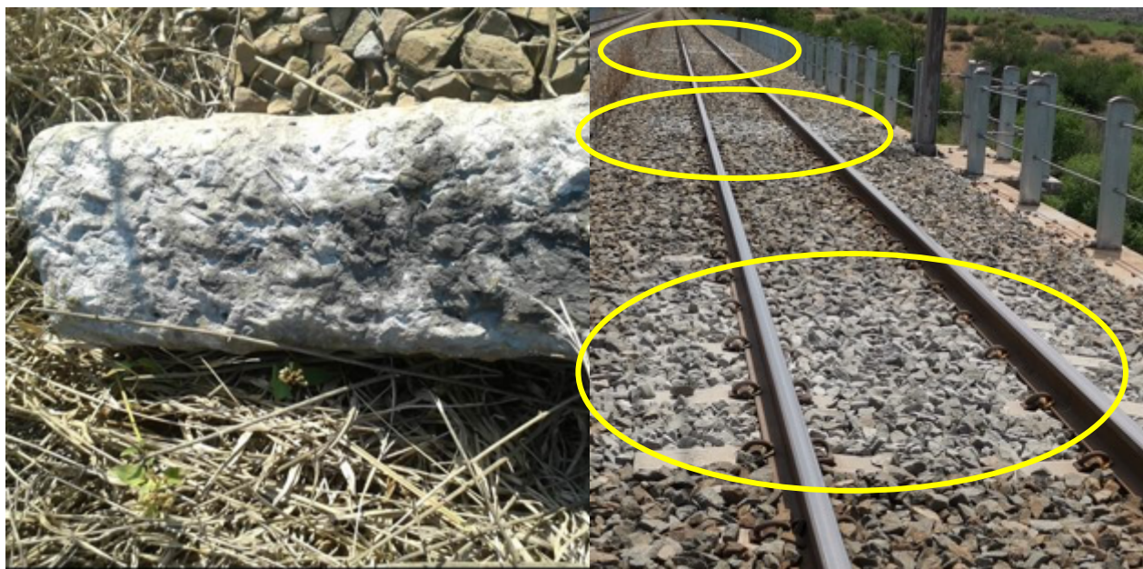
Figure 2-21: Sleeper Base Rounding due to abrasion near East London, Left; Localised Ballast/Sleeper abrasion and crushing near Kimberley, Right (Photos by Author).
