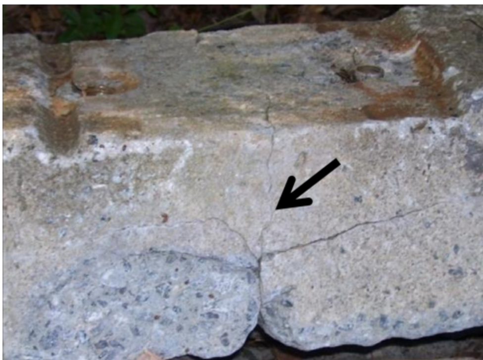
Figure 2-13: Example of a severe rail seat positive flexural crack (Zeman, 2010)
