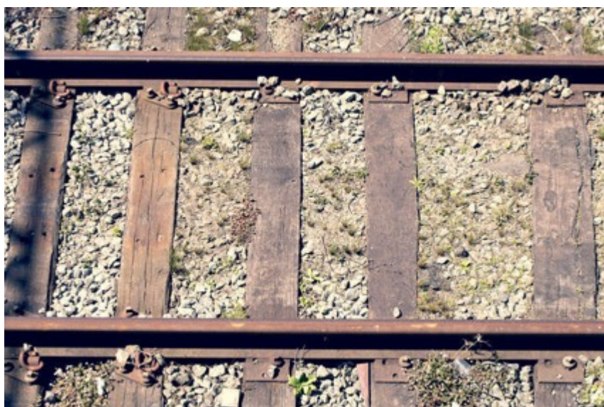
Figure 2-5: Example of Wooden Sleepers (Theos Timber Limited, 2017)
