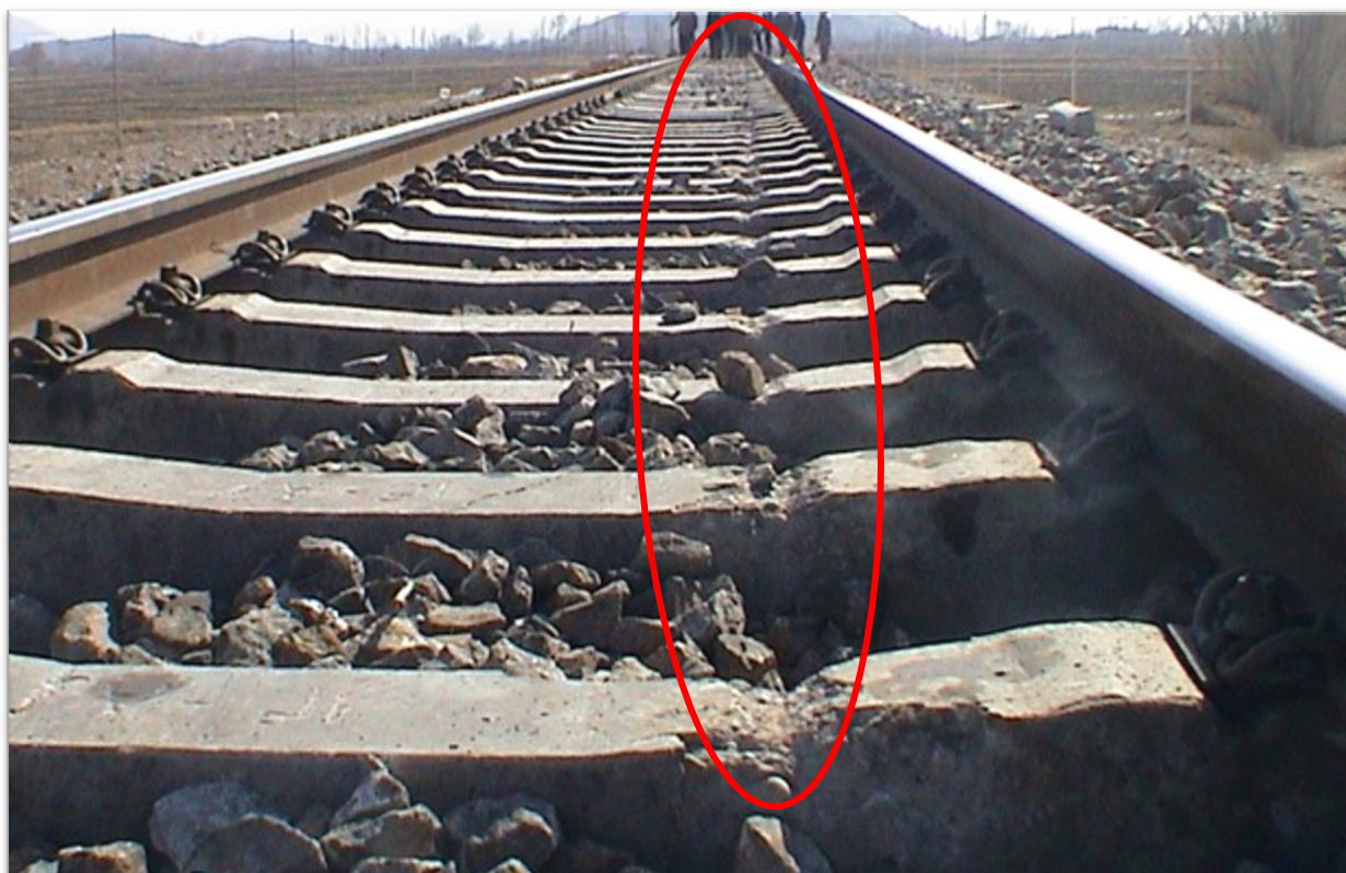
Figure 2-23: Derailment Damage from Wheel Dropping on the Gauge Side (Zakeri & Rezvani, 2012)
