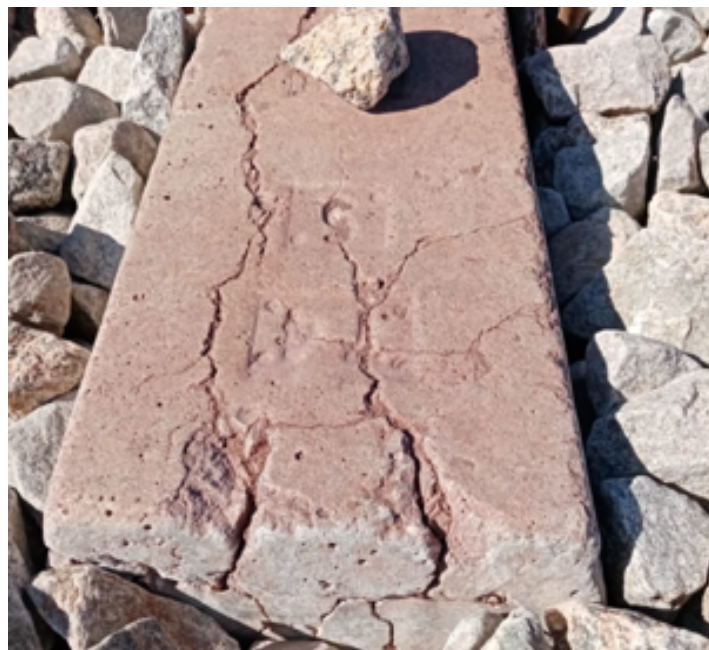
Figure 2-11: Examples of ASR Map Cracking from Sleeper Manufactured in 1974 in Saldanha PPC (Photo by Author)
