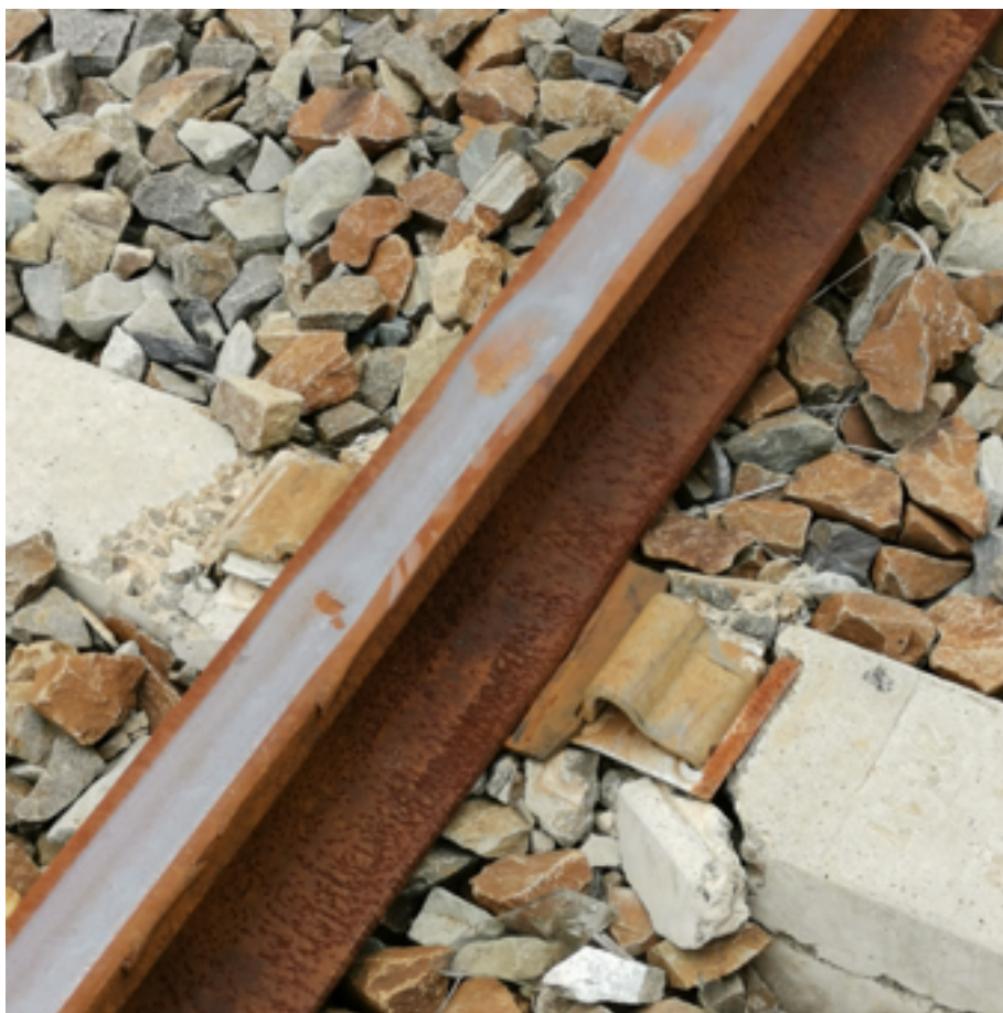
Figure 2-12: Sleeper Cracking under rail defect near East London (Picture by Author)
