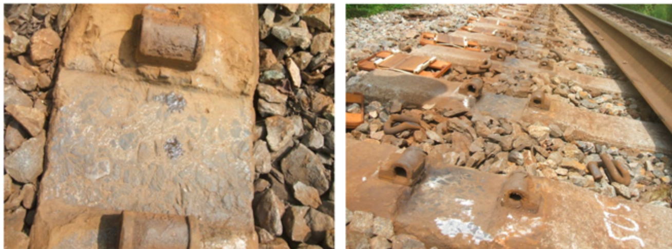
Figure 2-20: Typical Rail Seat Deterioration (RSD) (Federal Railroad Administration, 2019)
