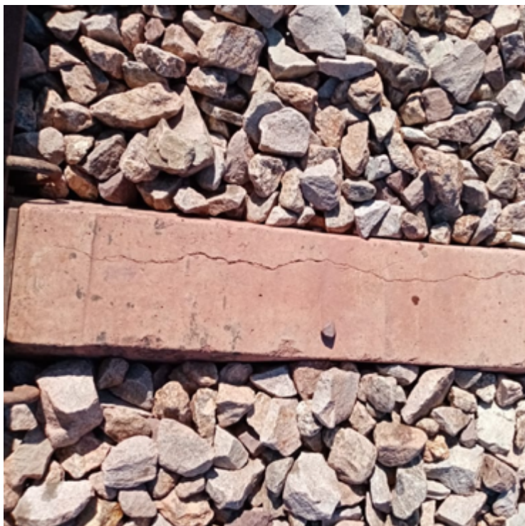
Figure 2-14: Long Horizontal Cracks on Sleeper in Northern Cape (Photo by Author)
