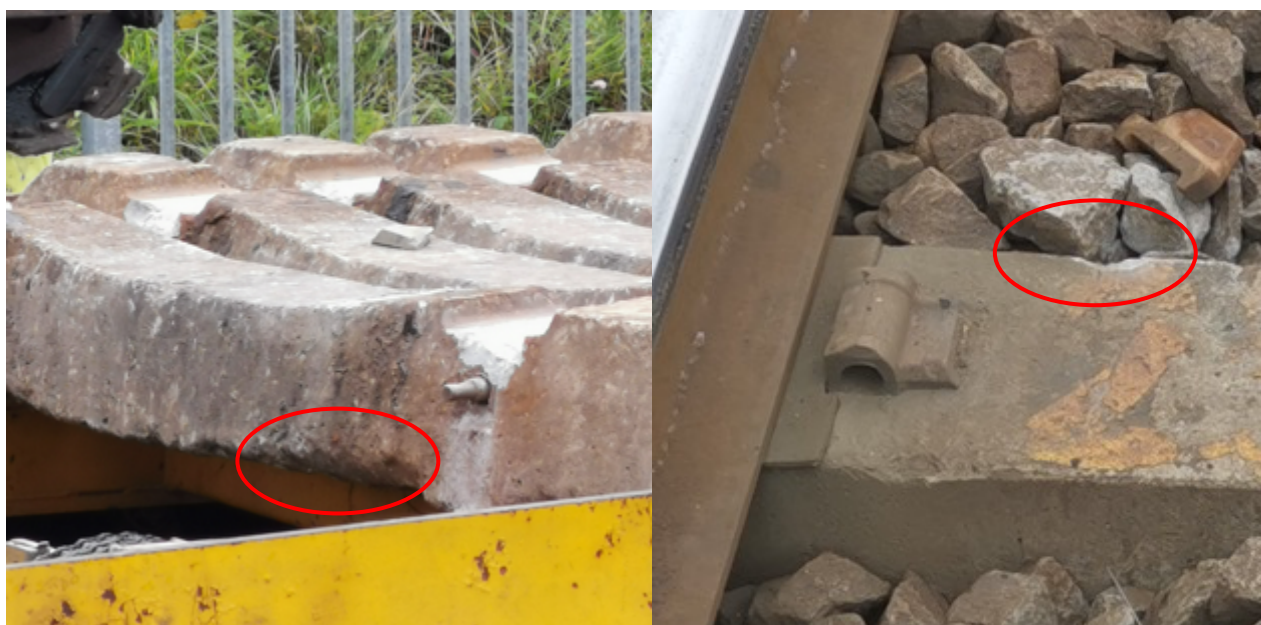
Figure 2-22: Base abrasion around rail seat due to Mechanized Ballast Tamping near East London, Left; Tamping Tine damage of sleeper near De Aar, Right. (Photos by Author)
