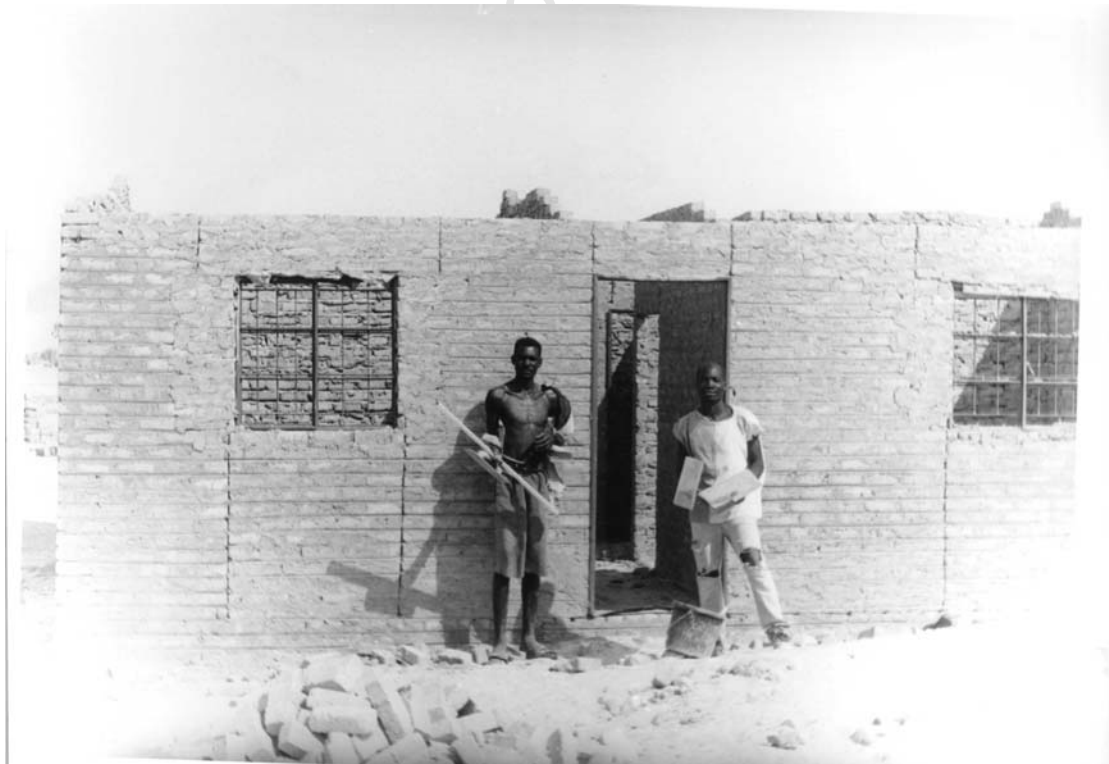
“This is one of the houses built through loans from the Build Together Programme in the informal settlements”. Photo 12: Magdalena Samuel
