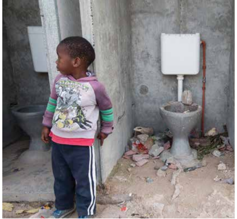
81: Child standing at the entrance of vandalised toilets.
