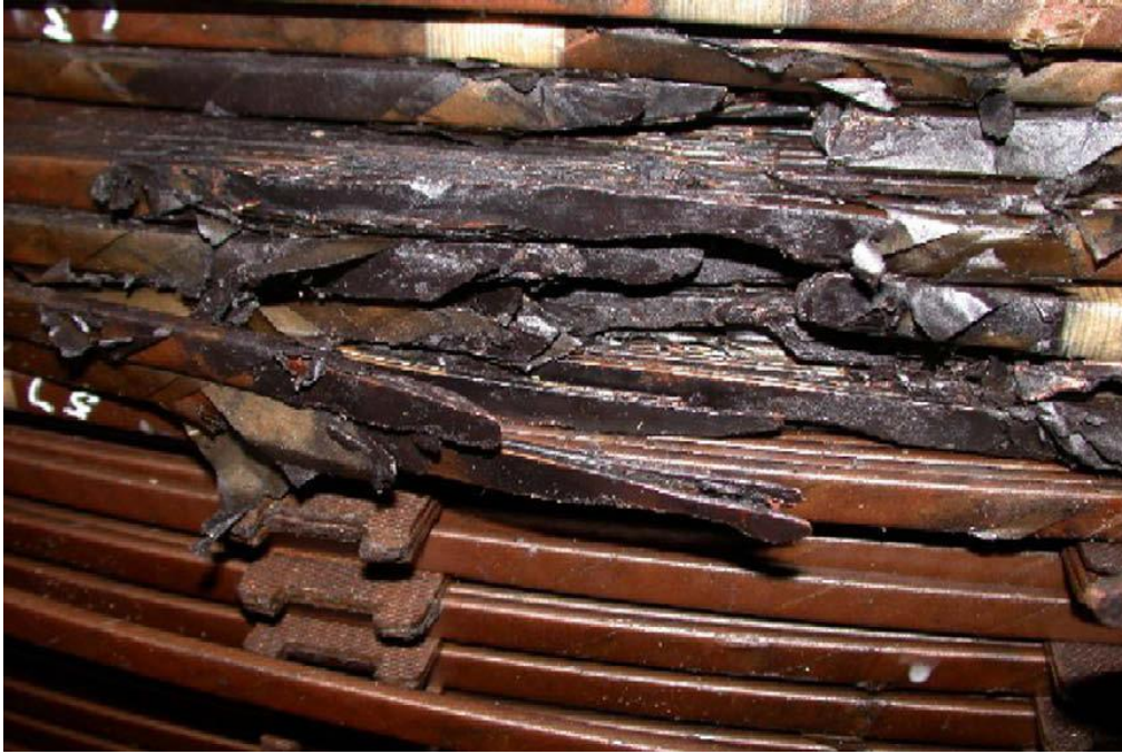
Figure 3: Disruption of the winding and insulation after initiation of damage during Halloween storm of October 2003 (Thomson et al. , 2010).
