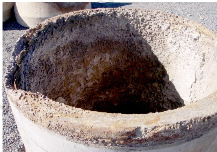
Figure 1.1 Deteriorated CAC/DOL sewer pipe concrete after 14 years of service at Virginia Experimental Sewer
