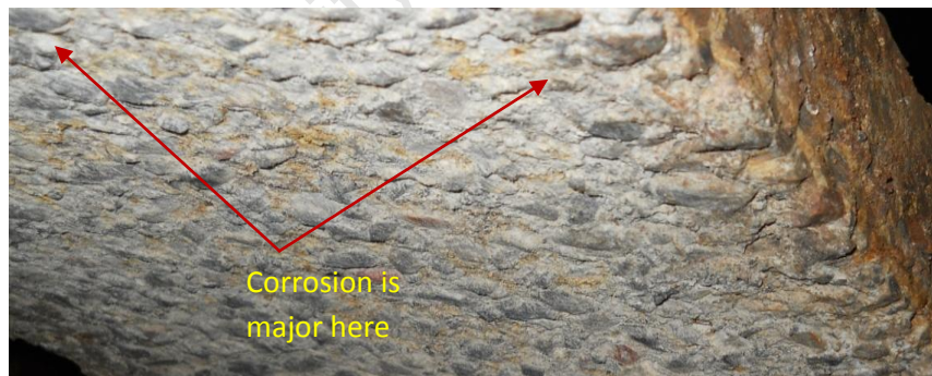
Figure 5.19 Moderate corrosion of OPC/FA/DOL concrete in Manhole III with aggregate particles clearly visible. Pipe sample was installed in October 2004.
