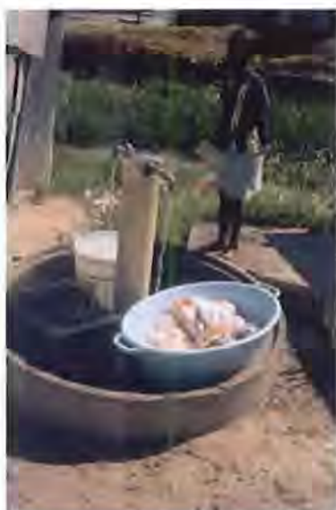
Figure B1.11: Tapstand at Khayelitsha RR (Sichone, 2006)
