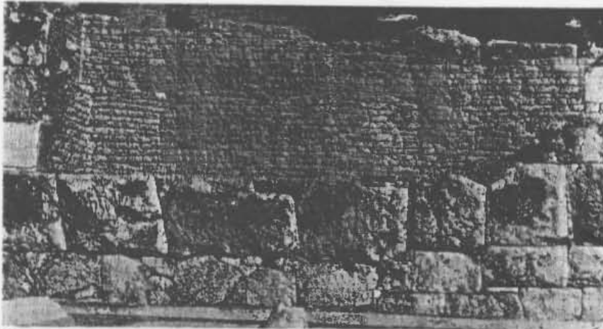
223 Section of the Themistoklean Wall west of the Sacred Gate, with repairs done by Conon and Demosthenes.
