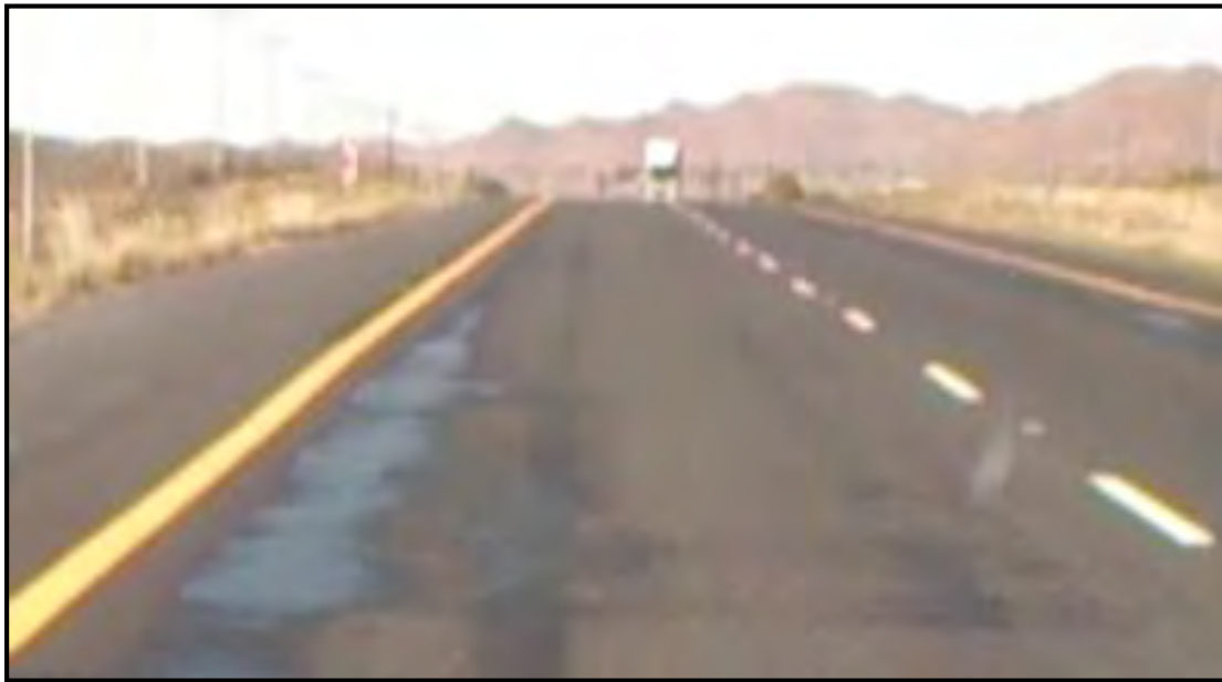
Figure 5.4: Road section affected by road surface bleeding
