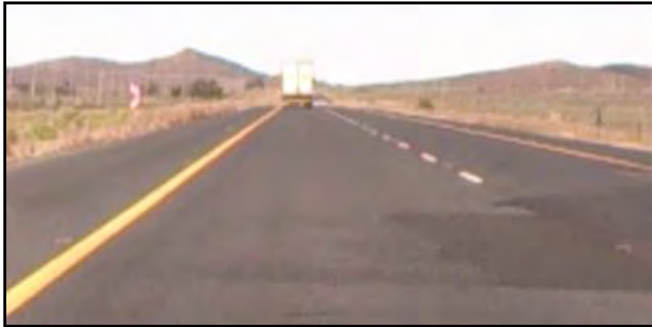
Figure 5.3: Obscured road marking on N1 highway
