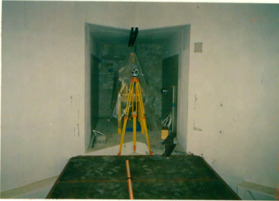
Figure 7.2. This photograph shows where the beam enters the treatment room. The precise level is being used to set out the floor.
