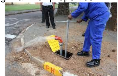
Figure 83: Fire hydrant should be maintained for reliable pressure during wildfire disaster
