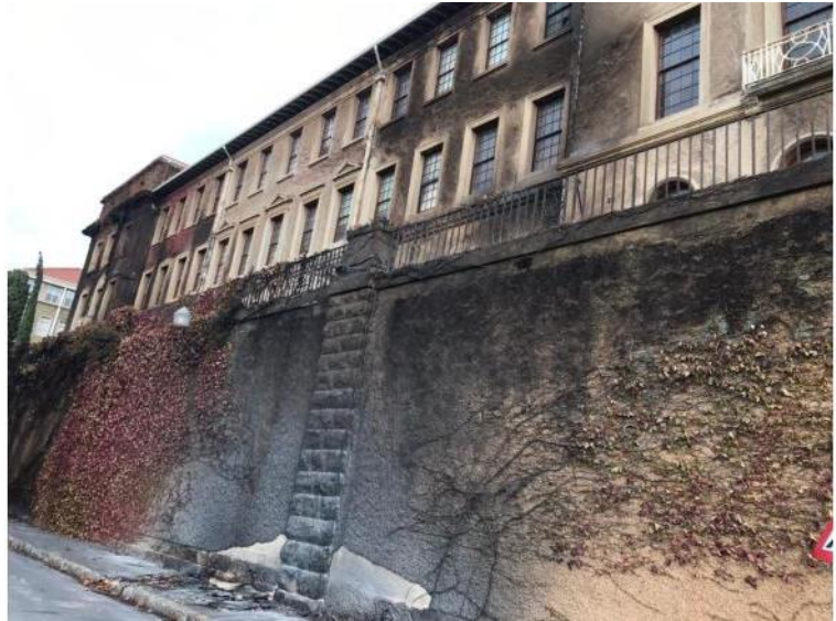
Figure 50: UCT creeping vines fire hazard (Charles, 2021).
