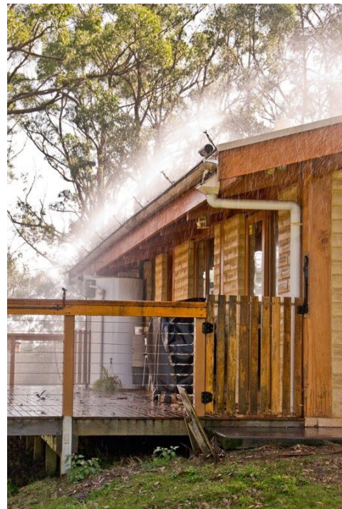
Figure 43: Installing burning ember protection system to a house, sprinklers on the roof (Terramatrix, 2020).
