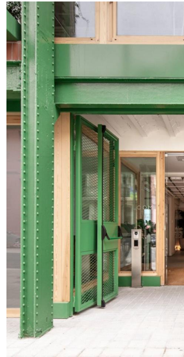
Figure 31 The entrance space into LOOM Coworking space. With the distinct green steelwork preserved and restored from the original building. (Jordi Bernardo, 2022)
