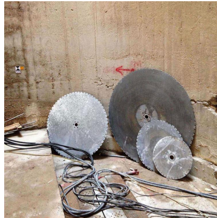
Figure 34 Zeitz MOCAA saw blades used to cut away the concrete silo tubes. (Heatherwick Studio, 2017)
