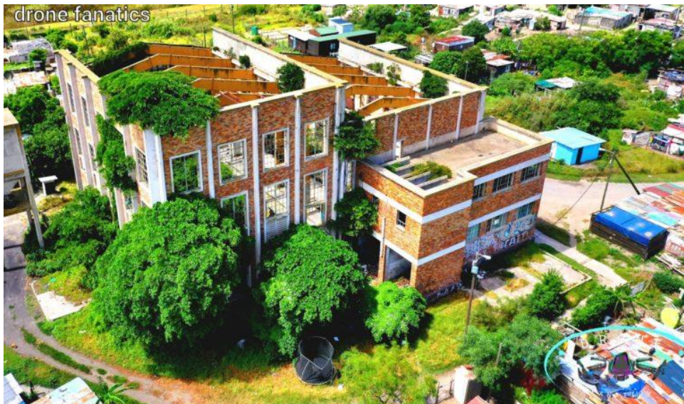
Figure 3 Kleinbrak abandoned power station, with natural reclamation occupying the insides. (Source Drone Fanatics 2022)
