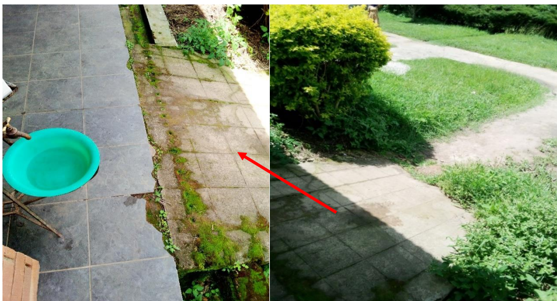
Figure 6.4: Walkway to the ANC clinic with a steep ramp and no handrails (Source: Field photo)
