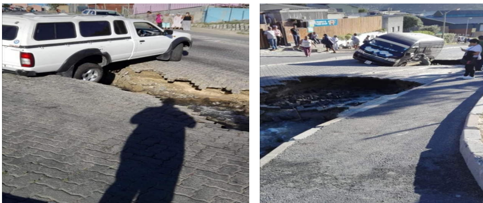
Figure 9: Showing Infrastructural decay. – Source Fieldwork pictures
