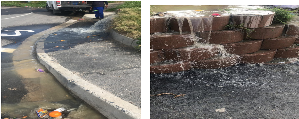
Figure 8: Picture showing sewage leaks and bursting pipes in Hangberg. Source - Fieldwork pictures
