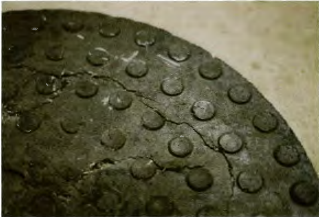
Figure 5.1.3. Crack propagation through to top surface of cover.
