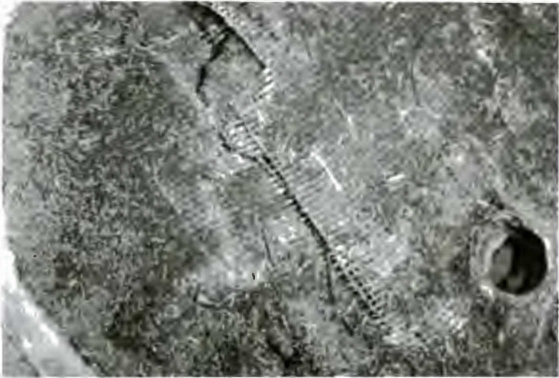
Figure 5.1.1 (c). Poor resin – mat adhesion (in this case accelerating failure).
