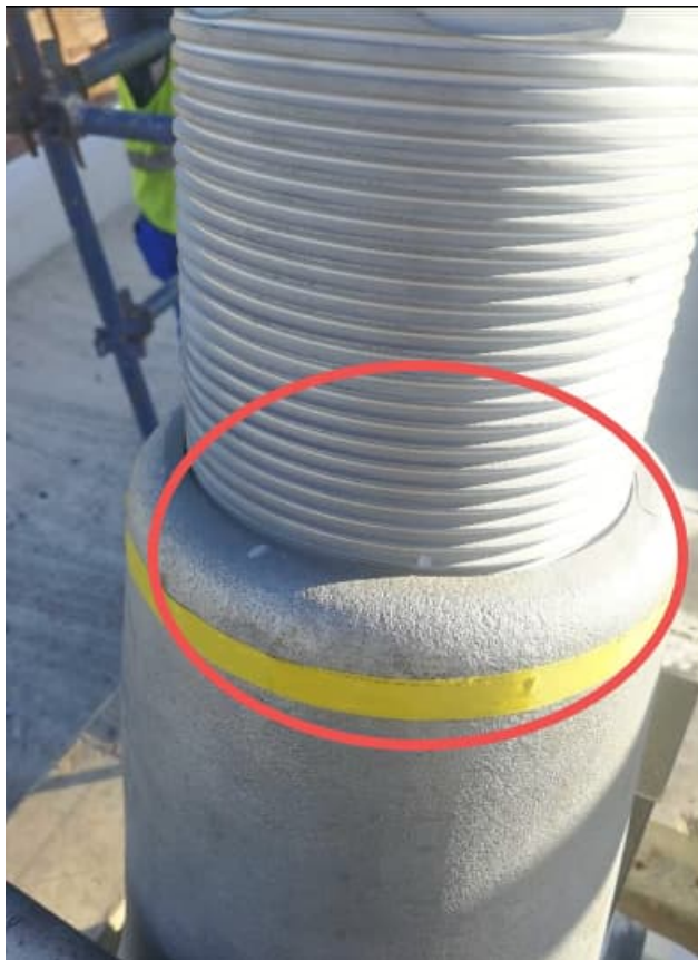
Figure 3-14: The gap measured between the two white marks after the turnbuckle was tightened
