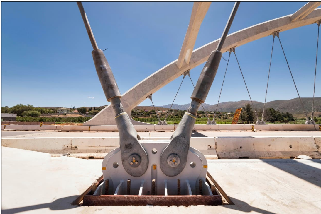
Figure 3-4: Connection between the adjustable fork socket and the cable. Photographed by Terry February for AECOM SA, 2020.
