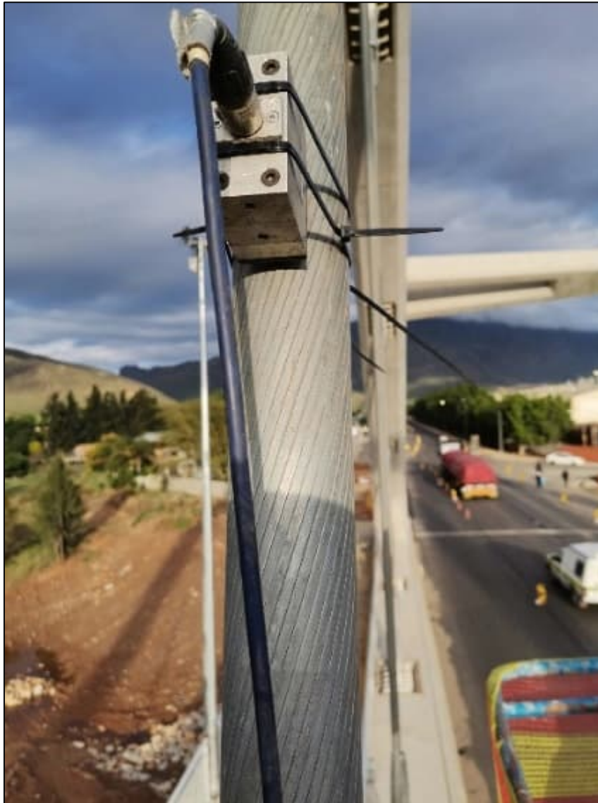
Figure 3-16: Accelerometer secured onto a cable
