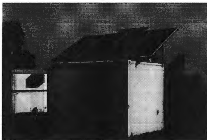
Figure 12: Eskom test hybrid system with container for storage of batteries, diesel generator, balance of system components and control, at Technology Research Institute, Eskom
