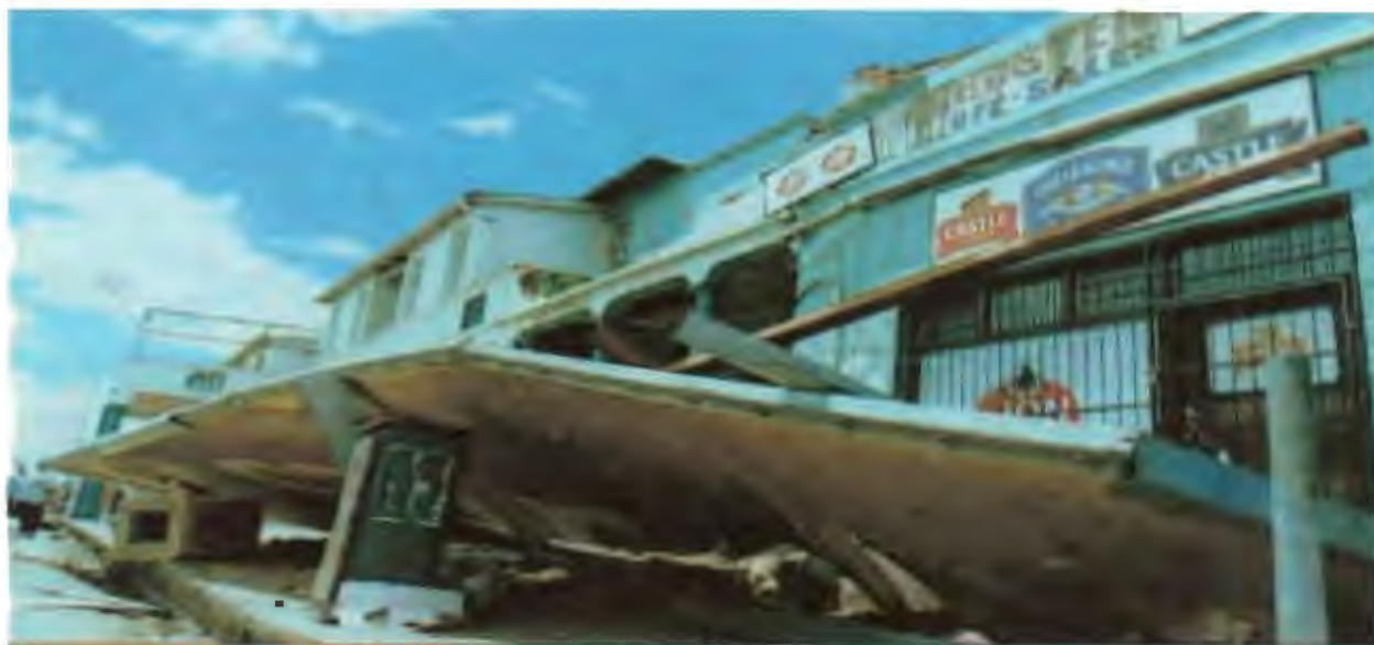
Figure 5.4. Evidence of the tornado damage in the city of Umtata located in Figure 5.3(b) as U.
