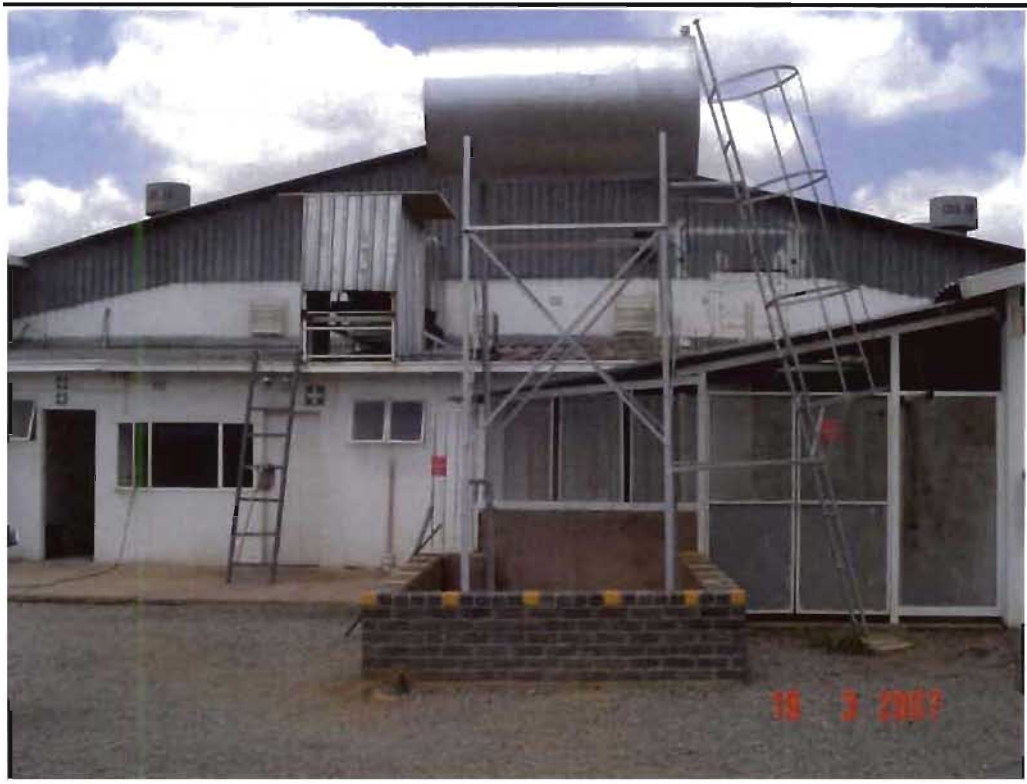
Photo 8.1 Site 1 - view of illuminating paraffin tank from 10m looking north
