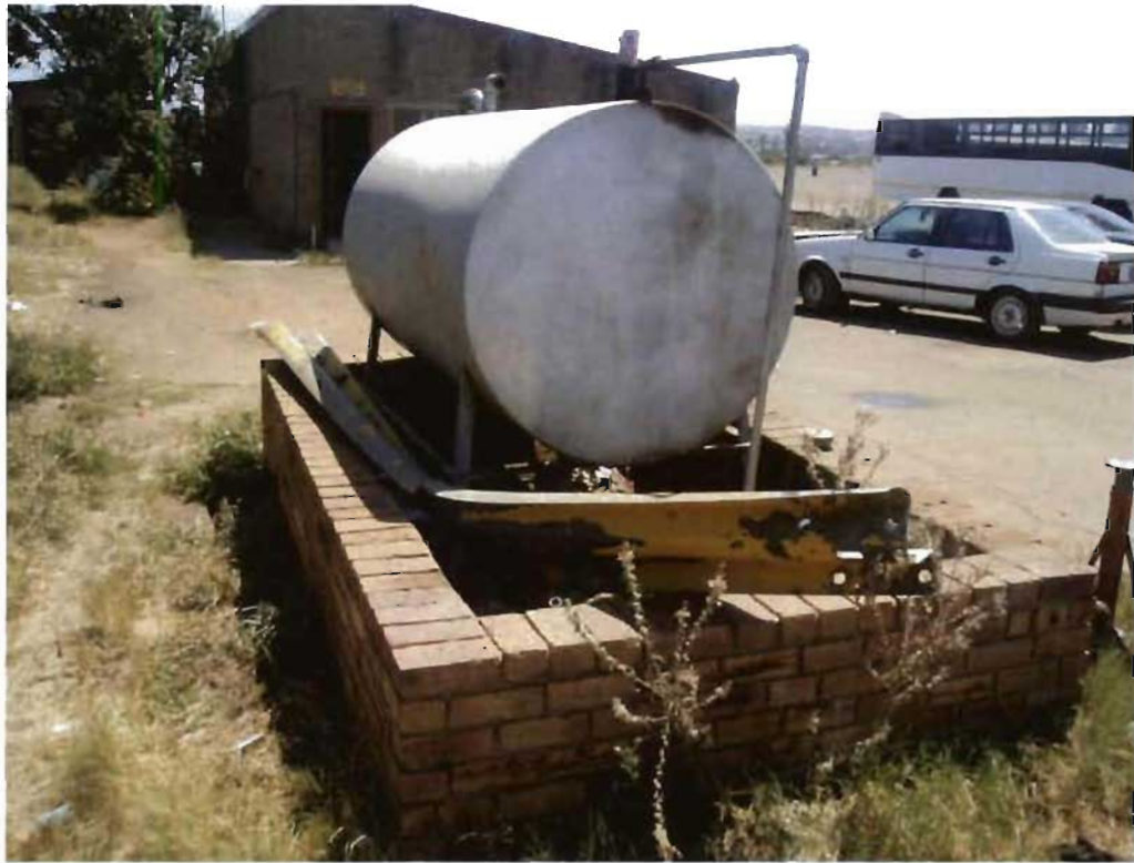
Photo 5.1 Location of tank 1 in relation to the depot offices looking north (S24/G/2/1023)
