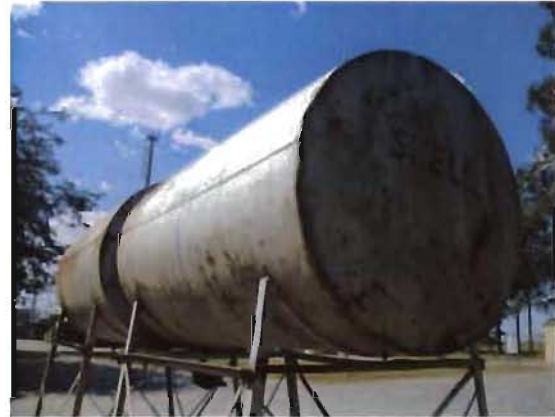
Fig. 3: Rust on Above-ground Tanks
