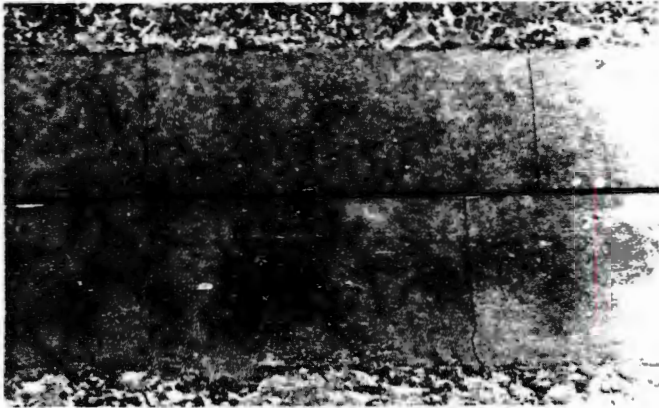
Fig 6: Transverse cracking of nosing as a result of curing shrinkage
