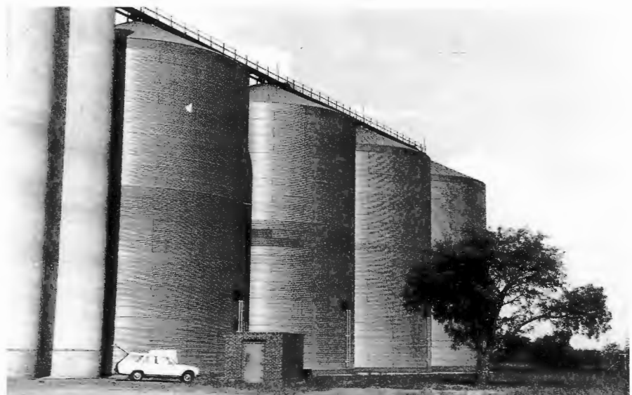
Fig. 1a: View of silo complex; test silo is on left closest to camera
