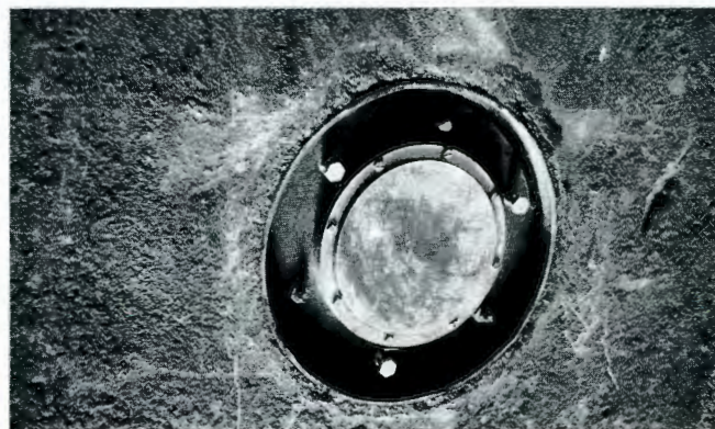
Fig. 3: View of pressure cell mounted in silo wall, before grouting and smoothing off flush with wall surface
