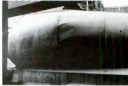
Fig. 8: 12.2 m diameter by 33 m high welded plane plate silo after collapsing and falling over as a result of eccentric emptying
