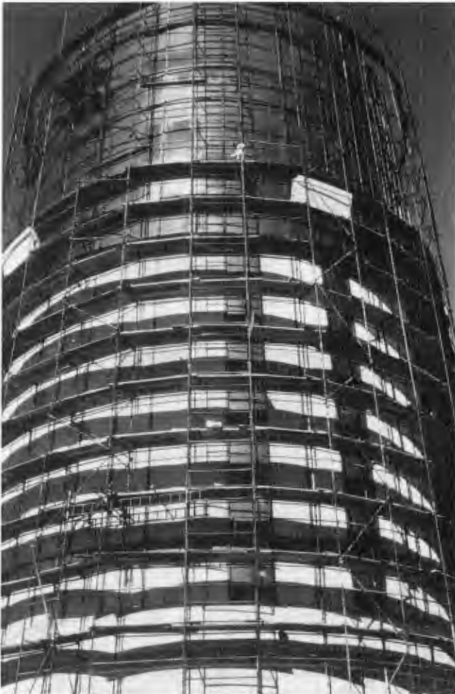
Fig. 6: View of silo while instrumentation was being installed (note man on tenth level of scaffolding)
