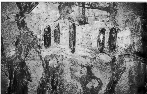
Fig. 7. Main reinforcing bars in column exposed: strain gauges mounted on second bar from right
