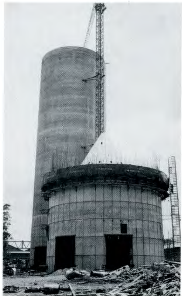
Figure 1. Silo 1 complete, pedestal to silo 2 complete with internal shuttering for cone in place.
