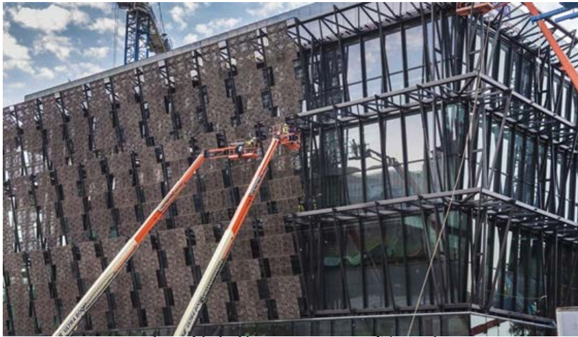
Figure 55: Construction phase of the building, image courtesy of The Smithsonian Institution and NMAAHC
