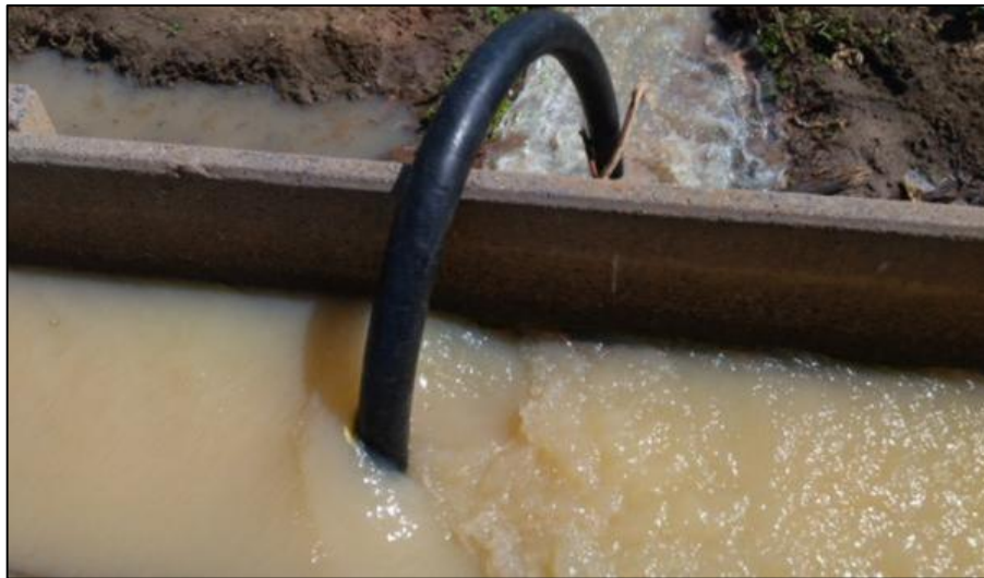
Figure 2-2: Water being siphoned from the parabolic canal to the farmland at Jibia Fadama Site.
