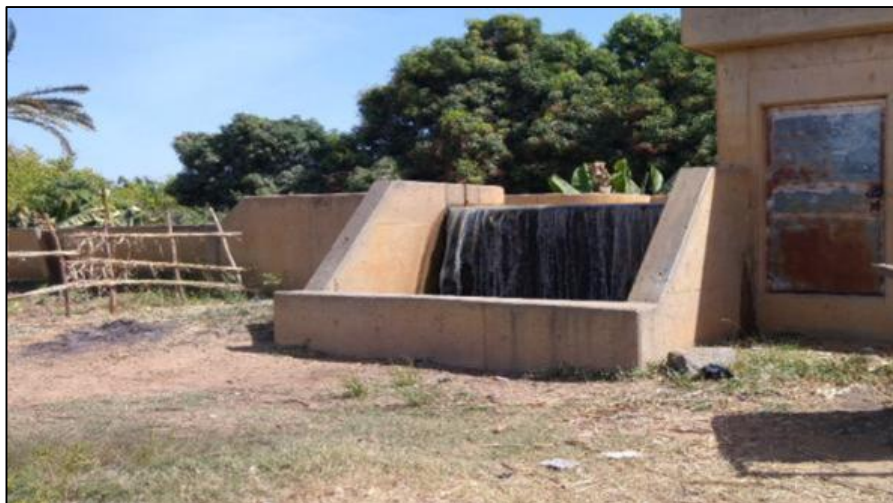
Figure 2-3: Water pumping station at Jibia dam, from this point water is further pushed to reach the canals around the Fadama field.
