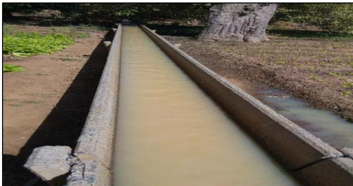
(a): Parabolic canal conveying water to the field. Jibia dam Fadama site.
