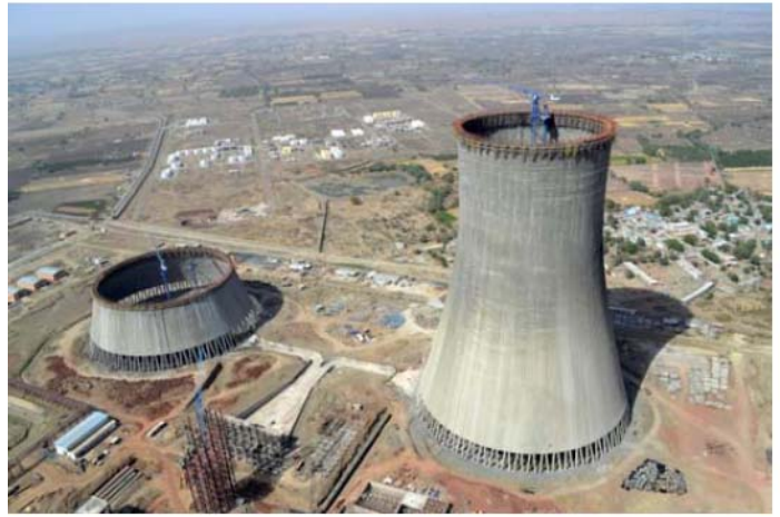
Figure 12: Construction of the Kalisindh cooling towers in Rajasthan (India) adopted from (Asadzadeh & Alam, 2014)
