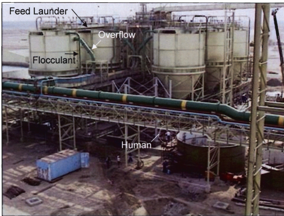
Figure 2.1 High compression thickeners (Bateman Ultrasep) at Orapa No. 2 Plant. Note the steep conical bases and the tall narrow cylindrical section. The feed is delivered to a central point via a launder, and then distributed to the thickeners.
