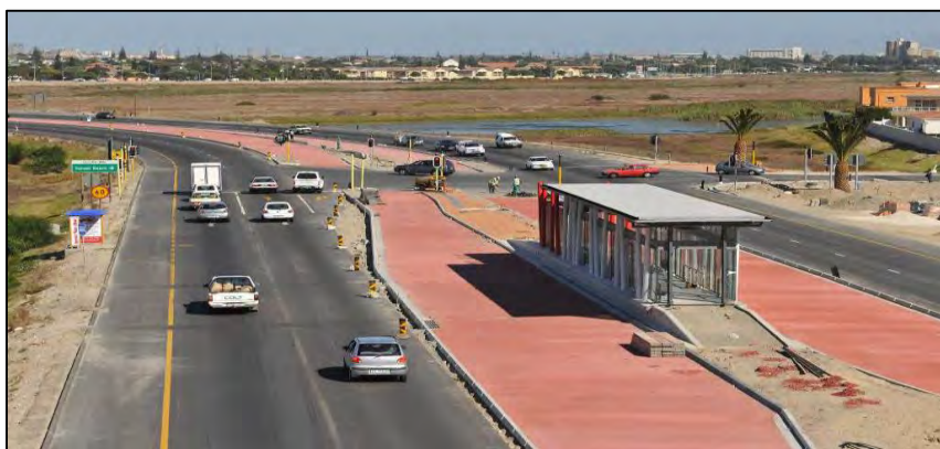
Figure 3-15 A section of Cape Town's BRT along the R27 during construction (CoCT,2012)
