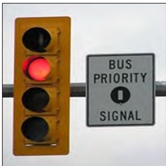
Figure 3-10 An Example a Bus Priority Signal Installation
